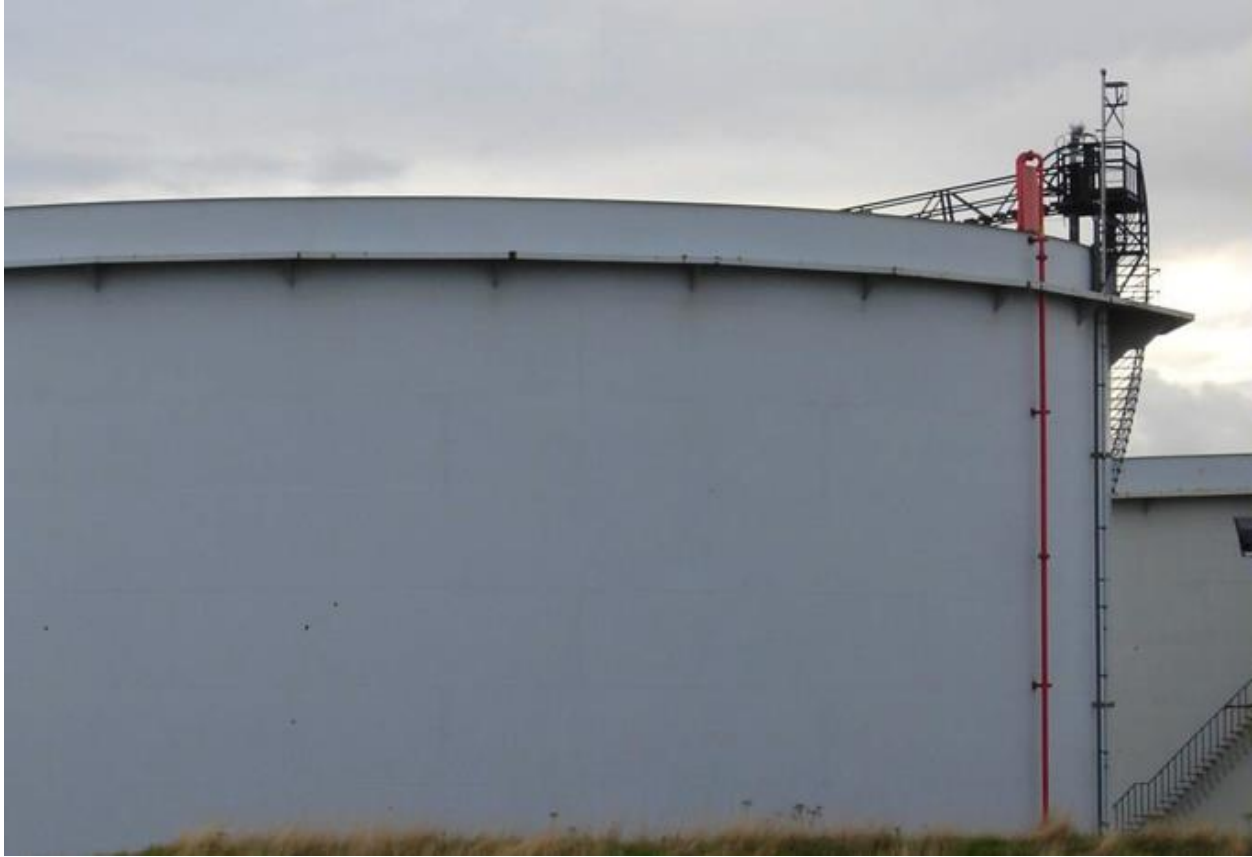
Figure 3 Overflow will impinge on wind girder and form a liquid cascade falling to the ground
