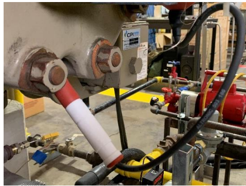
Figure 27: OC configuration on Ajax E-565 engine.
