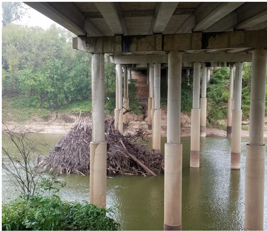
Figure 2.2 Woody debris accumulated against FM 60 (Raymond Stotzer Parkway) Overpass crossing the Brazos River (Photo Credit: Anita H. Brown)
