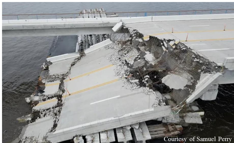
Figure 1.2 Damage to the Pensacola Bay (3 Mile) Bridge from Hurricane Sally (Robinson, 2020)
