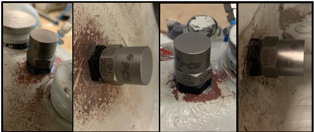
Figure 3.6: The four accelerometers attached to the GS-2 Terry Turbine.
