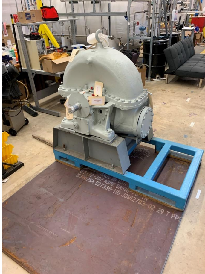
Figure 3.1: Photograph of the Clinton Power Station GS-2 Terry Turbine bolted to a steel pallet and resting on top of the steel working base.
