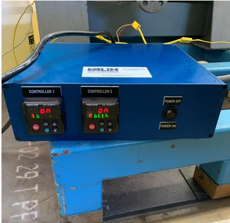
Figure 3.5: Valin Heater Control Console with power supplied connecting to Bluetooth connection.
