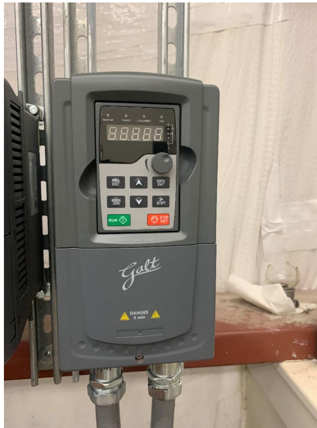
Figure 3.3: Variable frequency drive as installed in the laboratory.
