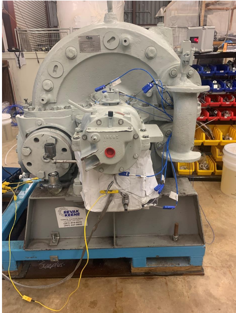
Figure 3.21: View of the Governor Side of the turbine with insulation on oil well and all instrumentation attached.
