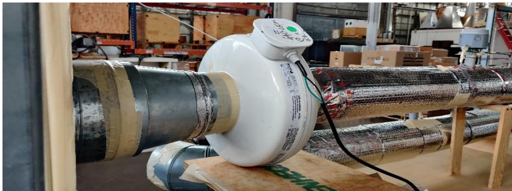
Figure 11 System of Dampers and Axial fans to regulate airflow in ducts
