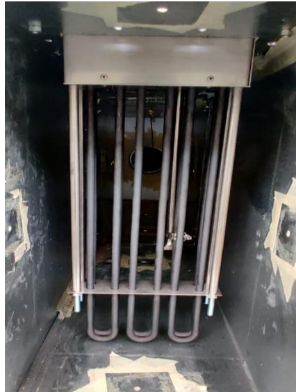
Figure 3 Heating coil in the rectangular duct
