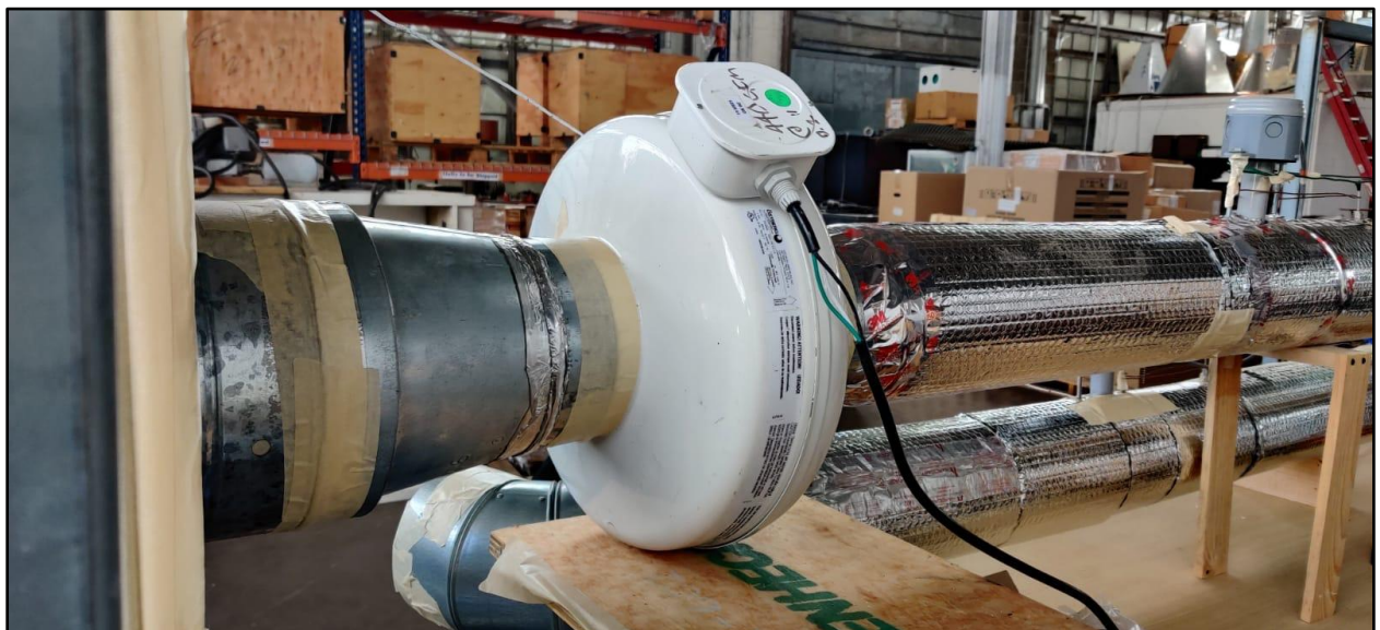
Figure 5. Inline fan installed at supply inlet
