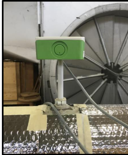
Figure 9. Air velocity transmitter installed in duct
