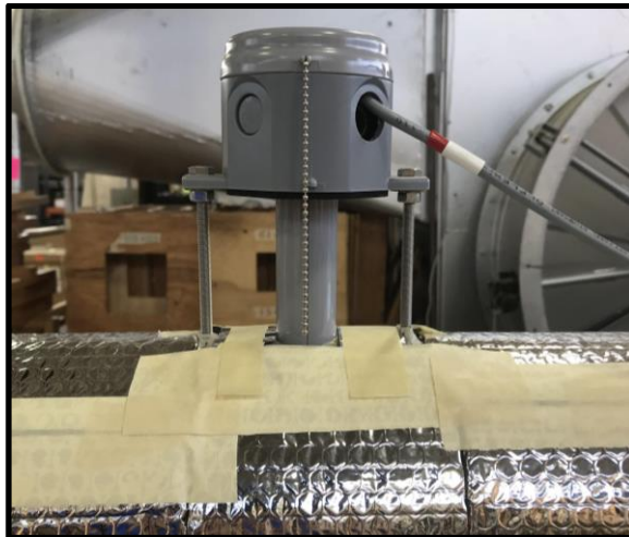
Figure 7. CO 2 and relative humidity sensor installed in duct
