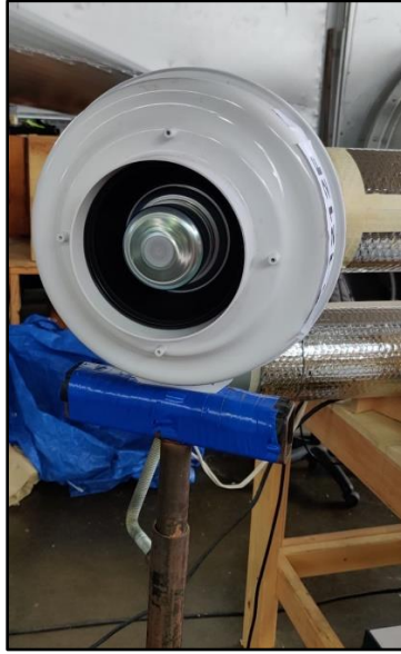
Figure 6. Inline fan installed at exhaust inlet
