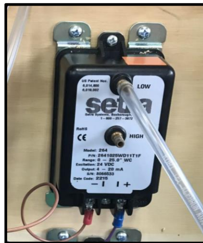
Figure 11. Pressure transducer connected to the test setup duct
