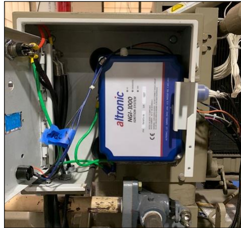
Figure 16: Altronic NGI-1000 ignition system installed on the Ajax E-565.
