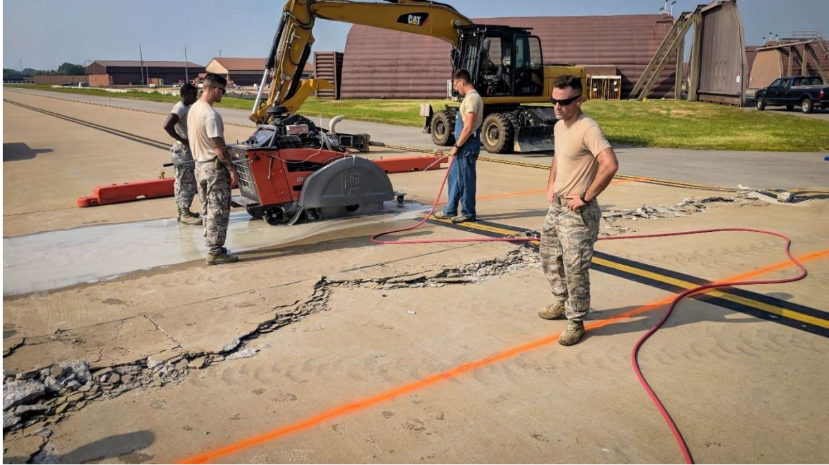
Figure 4. Taxiway Damage, Reprinted (Raughton, 2018)
