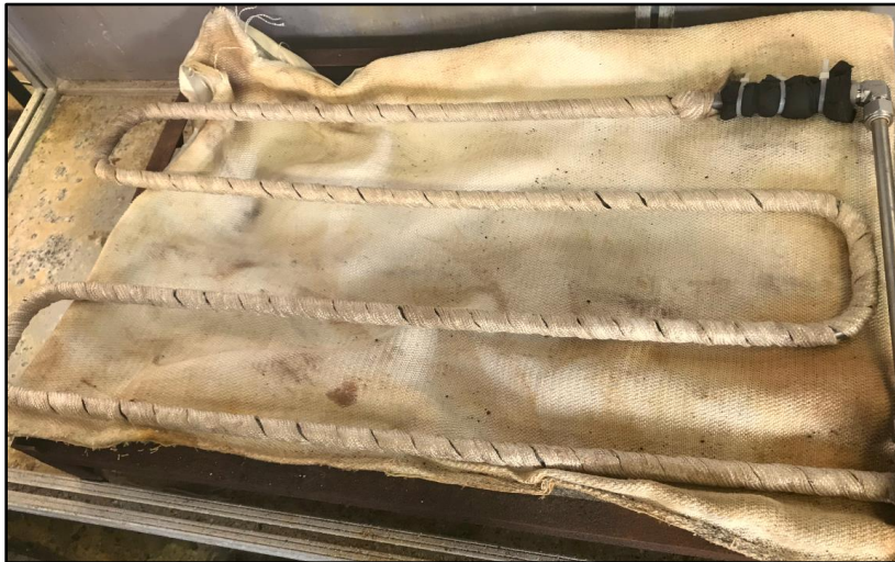
Figure 2-12: Heating tape to increase fluid temperature.
