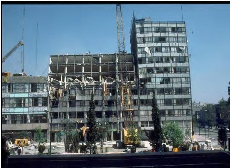
Figure 1-1 Pounding of adjacent buildings in Mexico City (1985) due to the SSI (Bisch et al., 2012)
