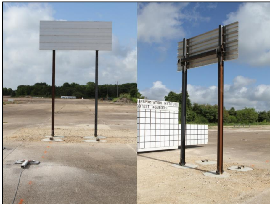
Figure 11. TxDOT W6x9 – 4-ft x 10ft Large Sign Support System (Reprinted from Silvestri et al., 2011)
