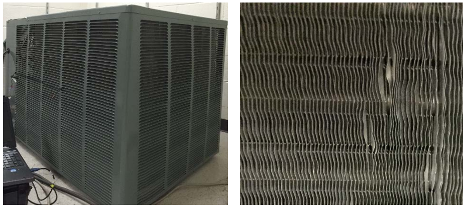
Figure 4-13 OD heat exchanger and fins.
