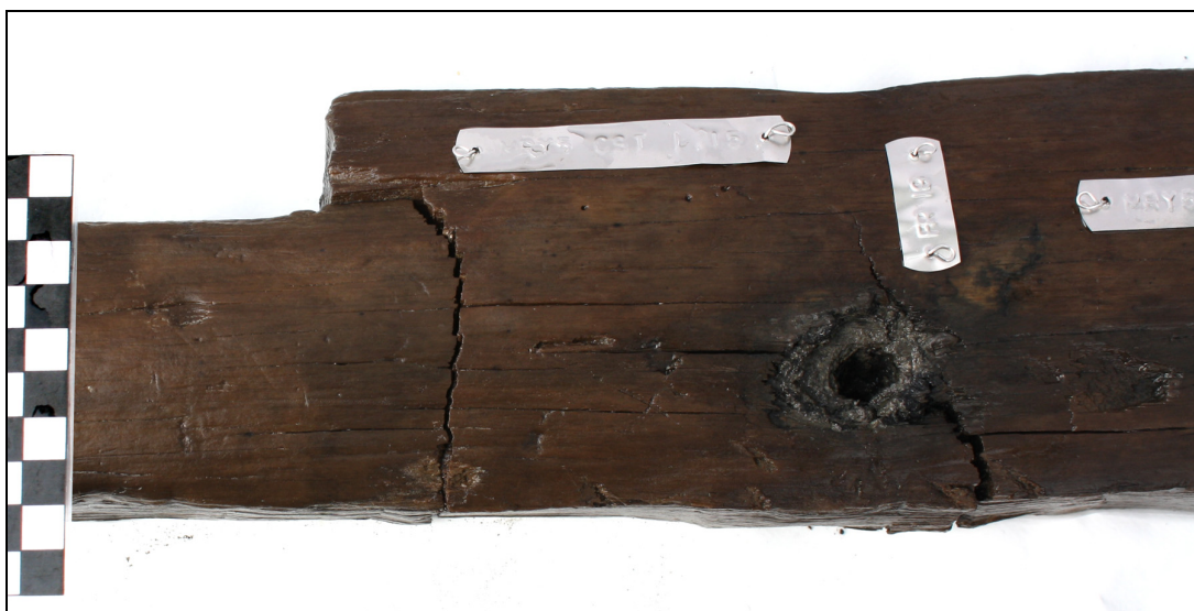
Figure 4.131. CST 1 inner face at FR 19. Note recess along inboard edge and deep pressure mark from nail head.
