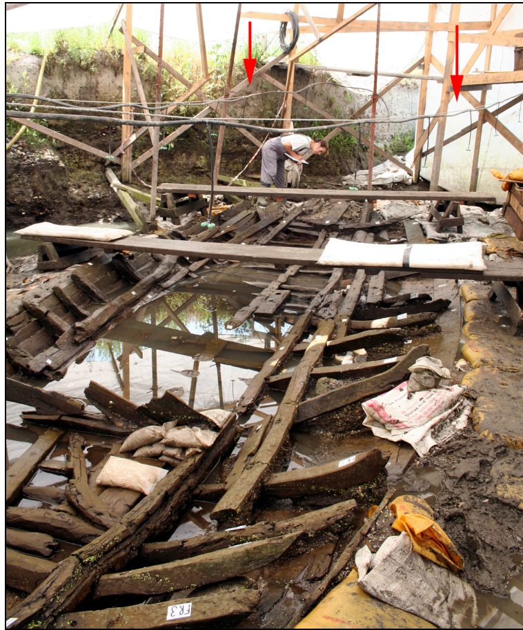
Figure 3.4. Shipwreck YK 11 during in-situ documentation. Two sprinkler lines (marked with red arrows) were installed above the wreck after it was uncovered. Long pallets, laid across sawhorses, provided access to the central part of the ship. June 21, 2008. Photo by R. Ingram/INA.
