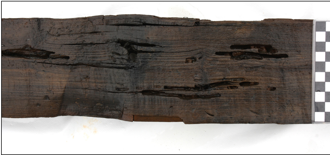
Fig. 4.135. Wood borer damage on the outer face of SST 4. Note saw marks and, at frame location, pressure damage.
