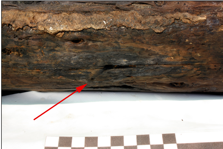
Figure 4.102. Outer face of SS 11 at FR 12. Note clenched nail tip (at arrow) and thick pitch and caulk near top edge.
