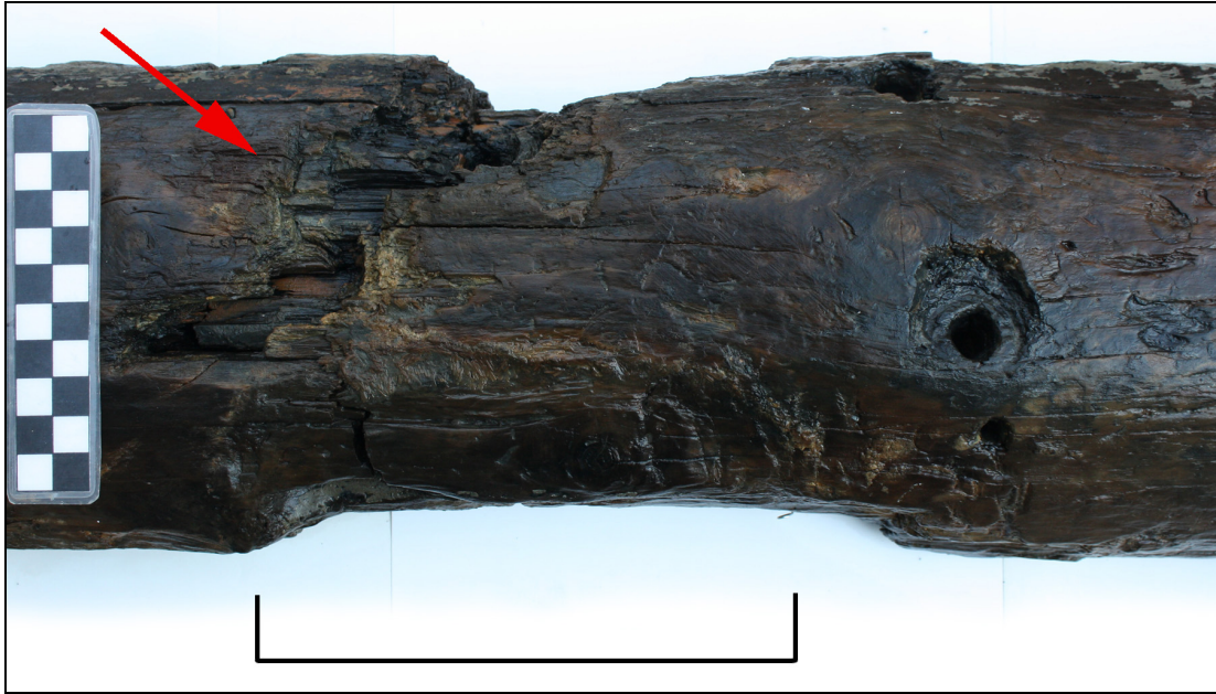
Figure 4.107. SS 13 outer face at FR 10-FR 11. Red arrow indicates rough tool marks that had been pitched over. Note pressure mark and caulk outline at through-beam location (indicated in black).
