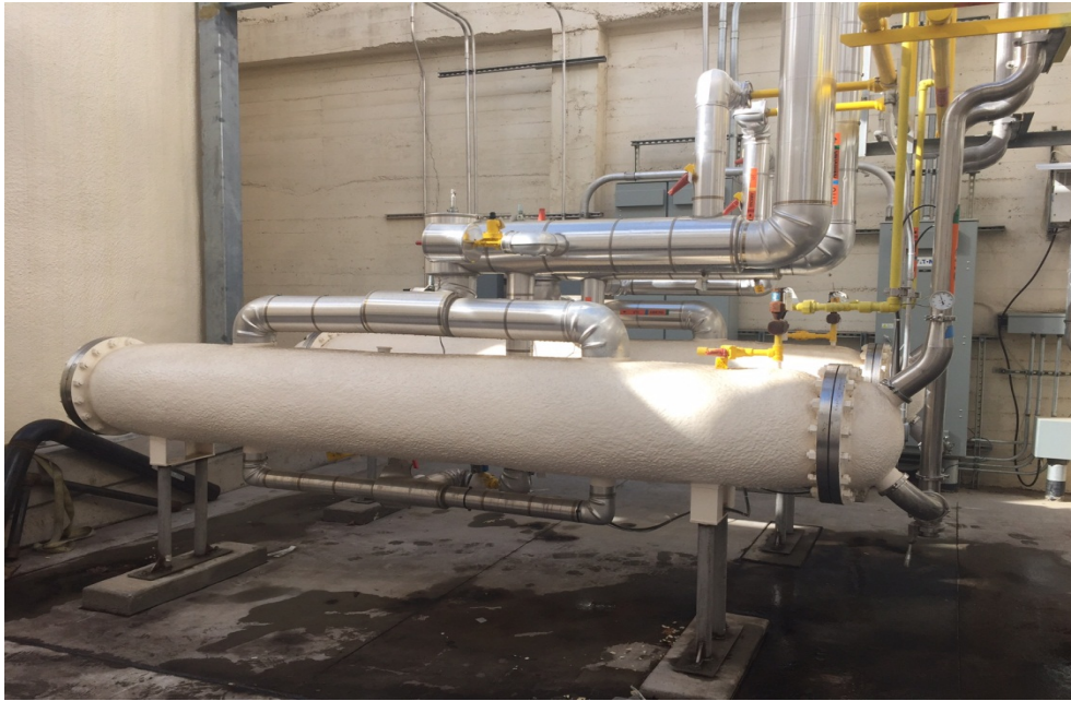
Fig 2.19: SX Chiller installed at California Wine Plant
