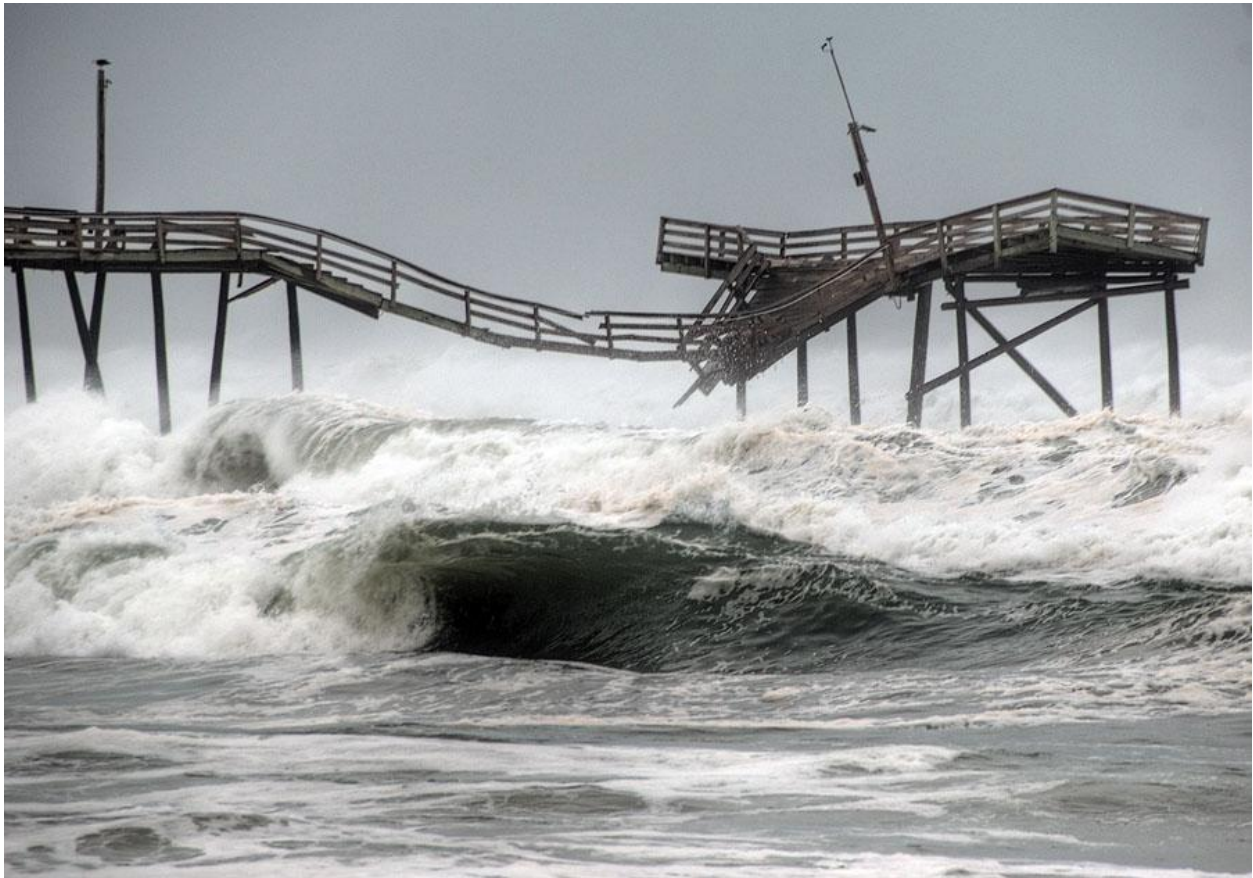
Figure 2: Pier destruction after hurricane
