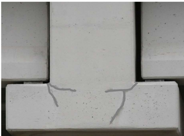
(a) Cracks on inverted-T bent cap in Austin, Texas
