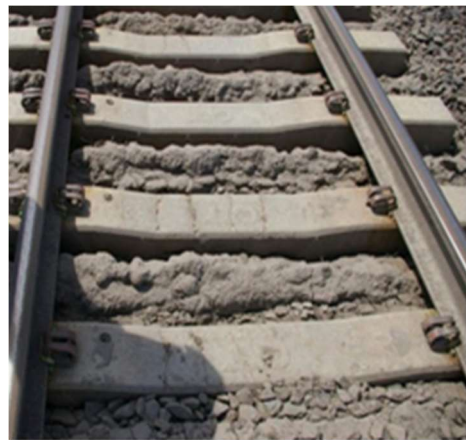
(b) Crack on concrete railroad ties. Reprinted from [1]
