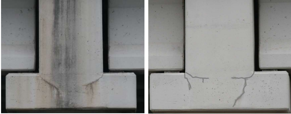
(a) Cracks on two bent caps near Austin, Texas. (crack highlighted)
