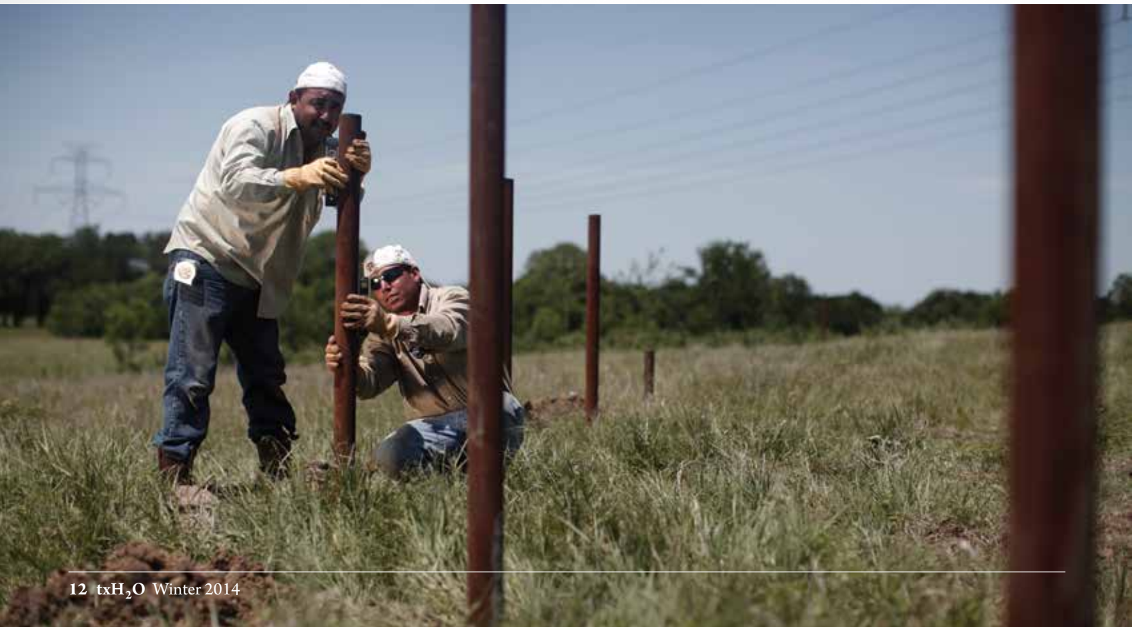
Workers install a fence on the 77 Ranch as part of Water As A Crop’s cost-share program to promote sustainable land management. Photo by Craig Ficenec, Water As A Crop.
