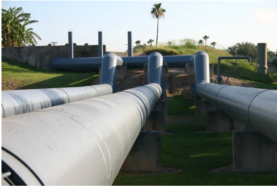
Pumping station on the Rio Grande
