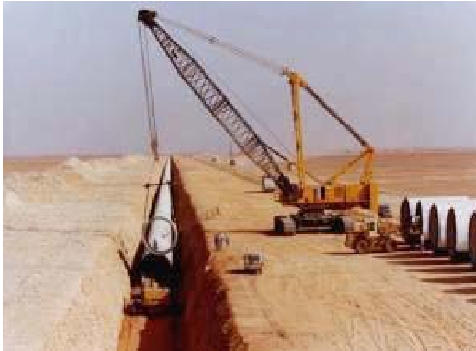
Figure 7: Example of underground pipe
