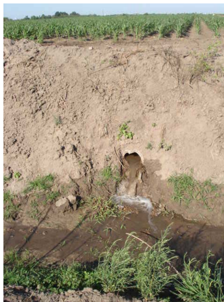
Figure 3. Irrigation return flows from a sub-surface drain flowing into a drainage canal
