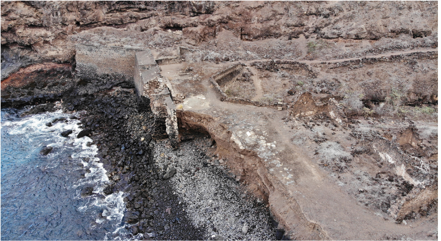
Figure 19: Aerial image of failing curtain wall looking north Lower Banks' Battery (Image: B. Fortenberry).
