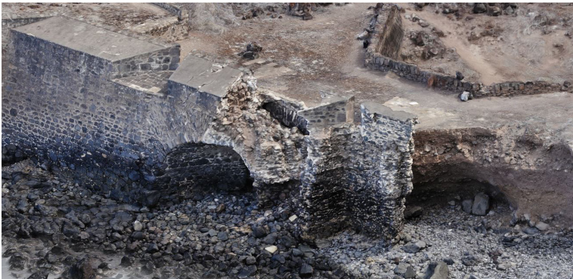
Figure 10: Photogrammetric model, arch collapse detail at Lower Banks' Battery (Model: B. Fortenberry).
