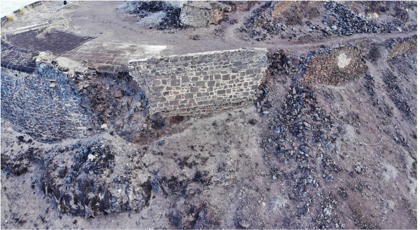
Figure 40: Oblique aerial view of wall collapse at Upper Banks' Half Moon Battery (Image: B. Fortenberry).
