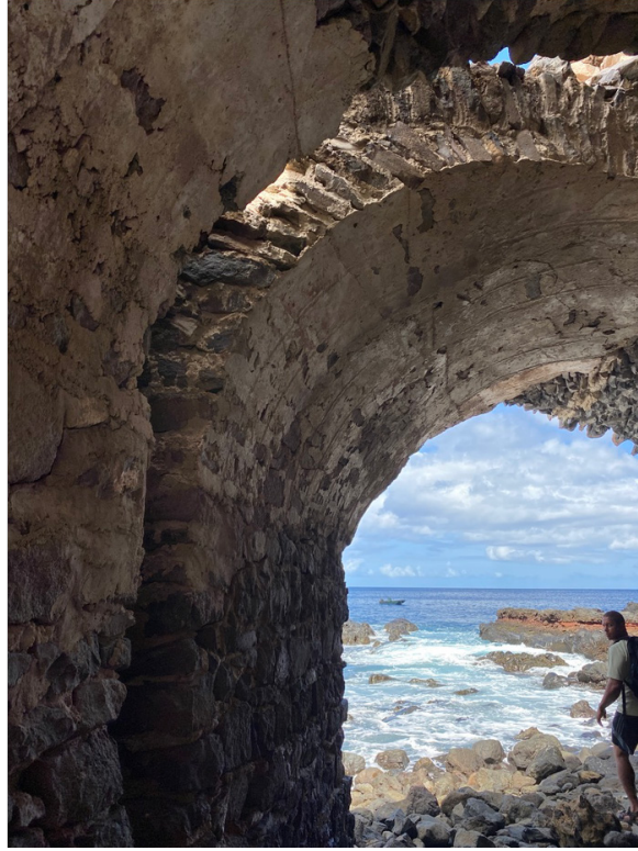
Figure 33: Detail of failing arch at Lower Banks' Battery (Image: B. Fortenberry).
