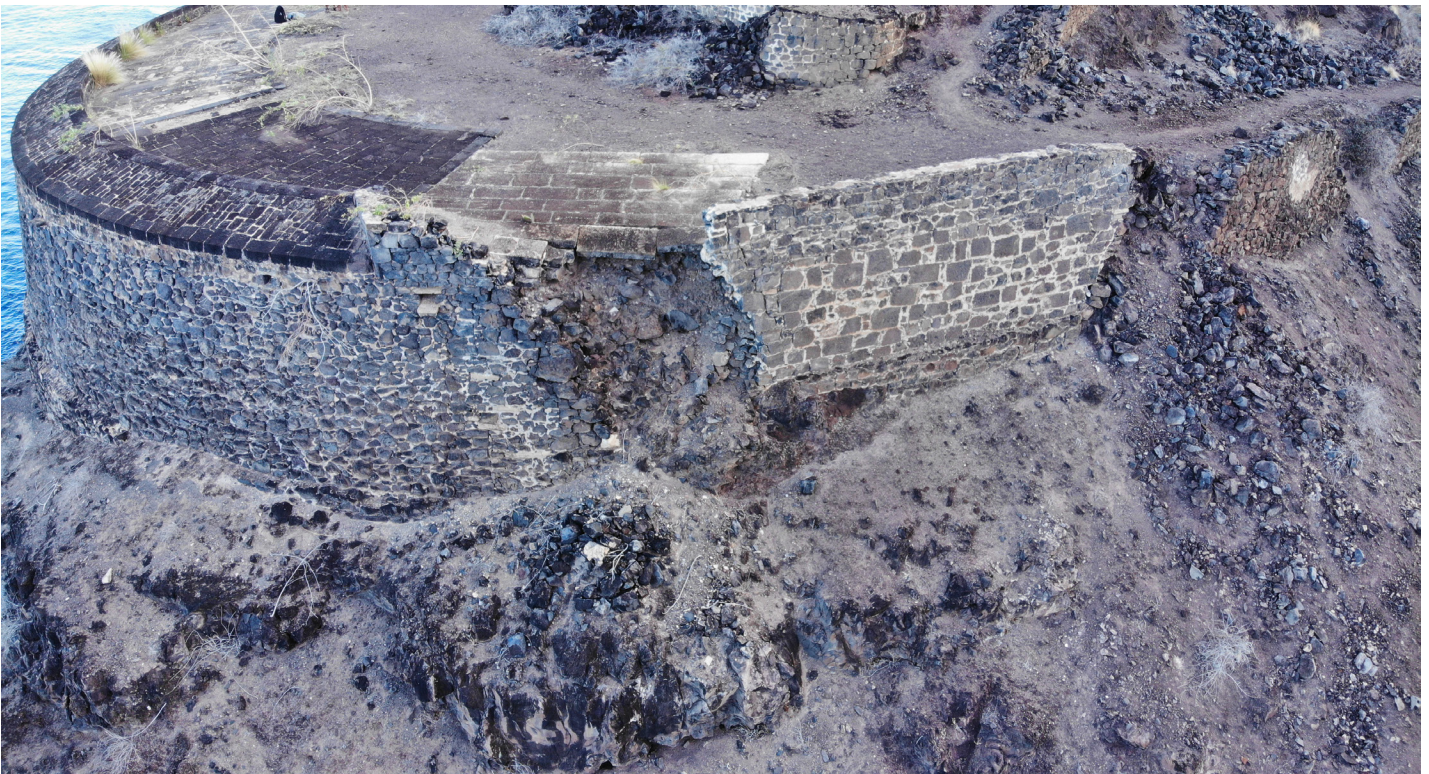
Figure 41: Oblique aerial view of wall collapse at Upper Banks' Half Moon Battery (Image: B. Fortenberry).
