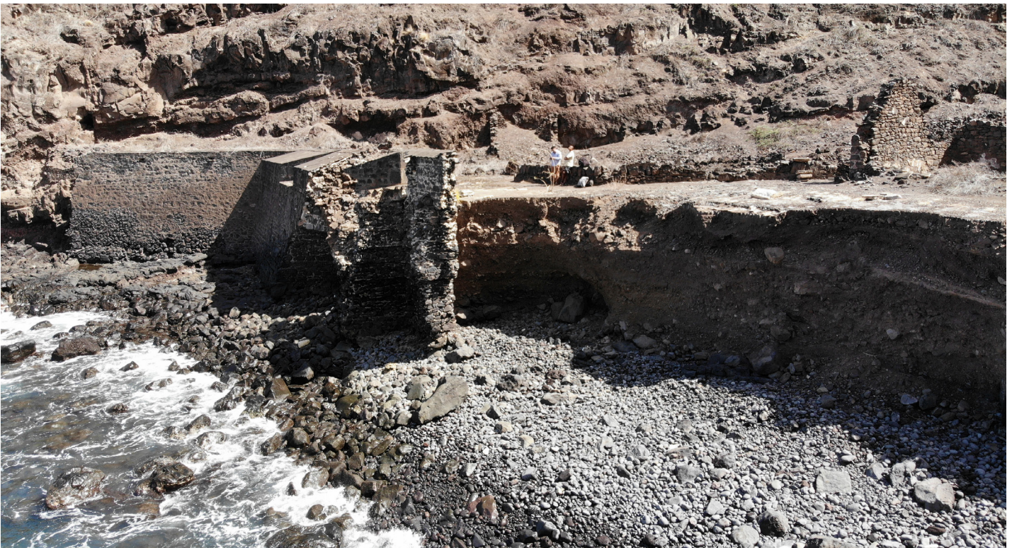
Figure 28: Aerial section image of failing curtain wall at Lower Banks' Battery (Image: B. Fortenberry).
