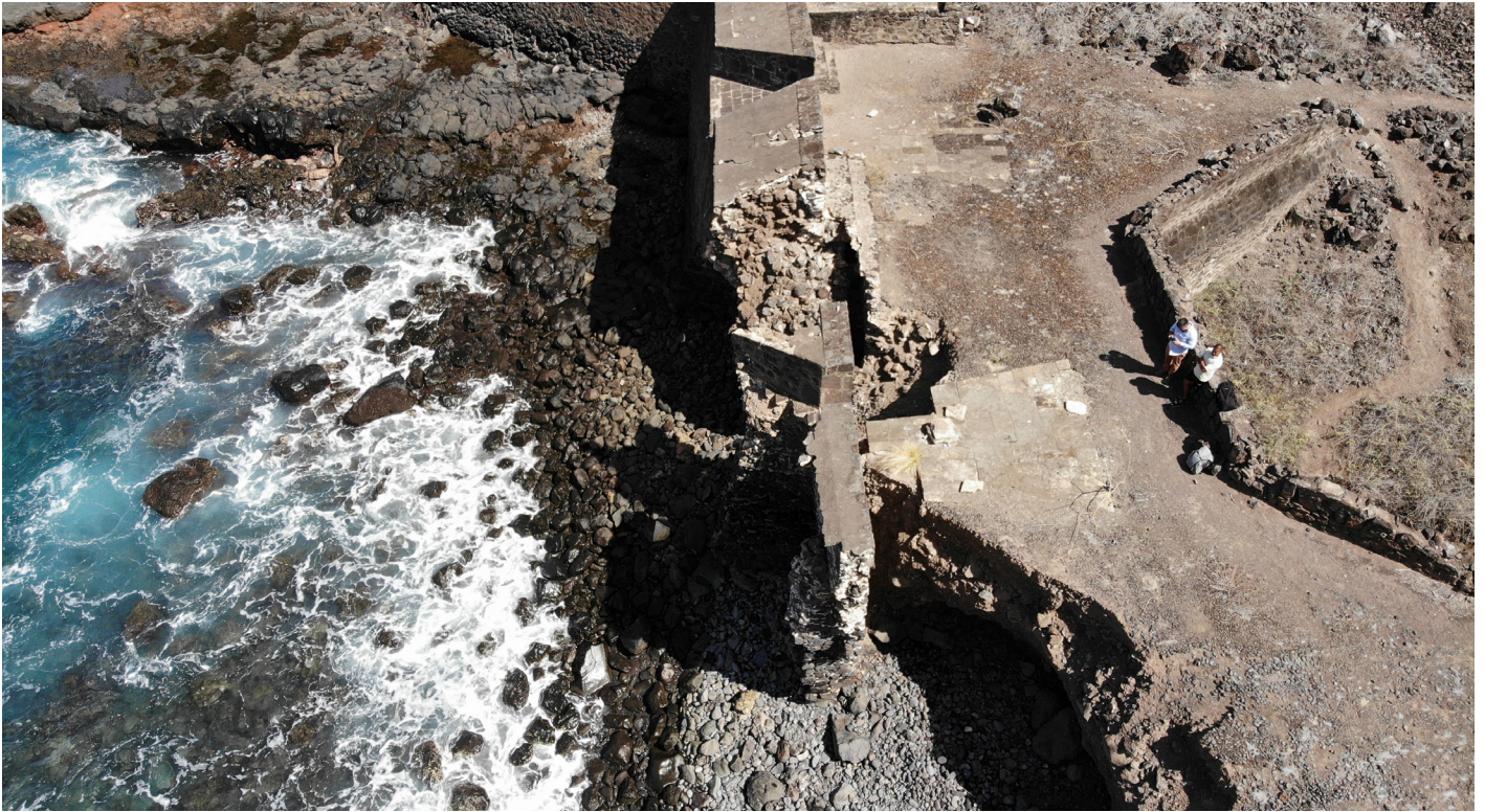
Figure 29: Aerial oblique image of failing curtain wall at Lower Banks' Battery (Image: B. Fortenberry).
