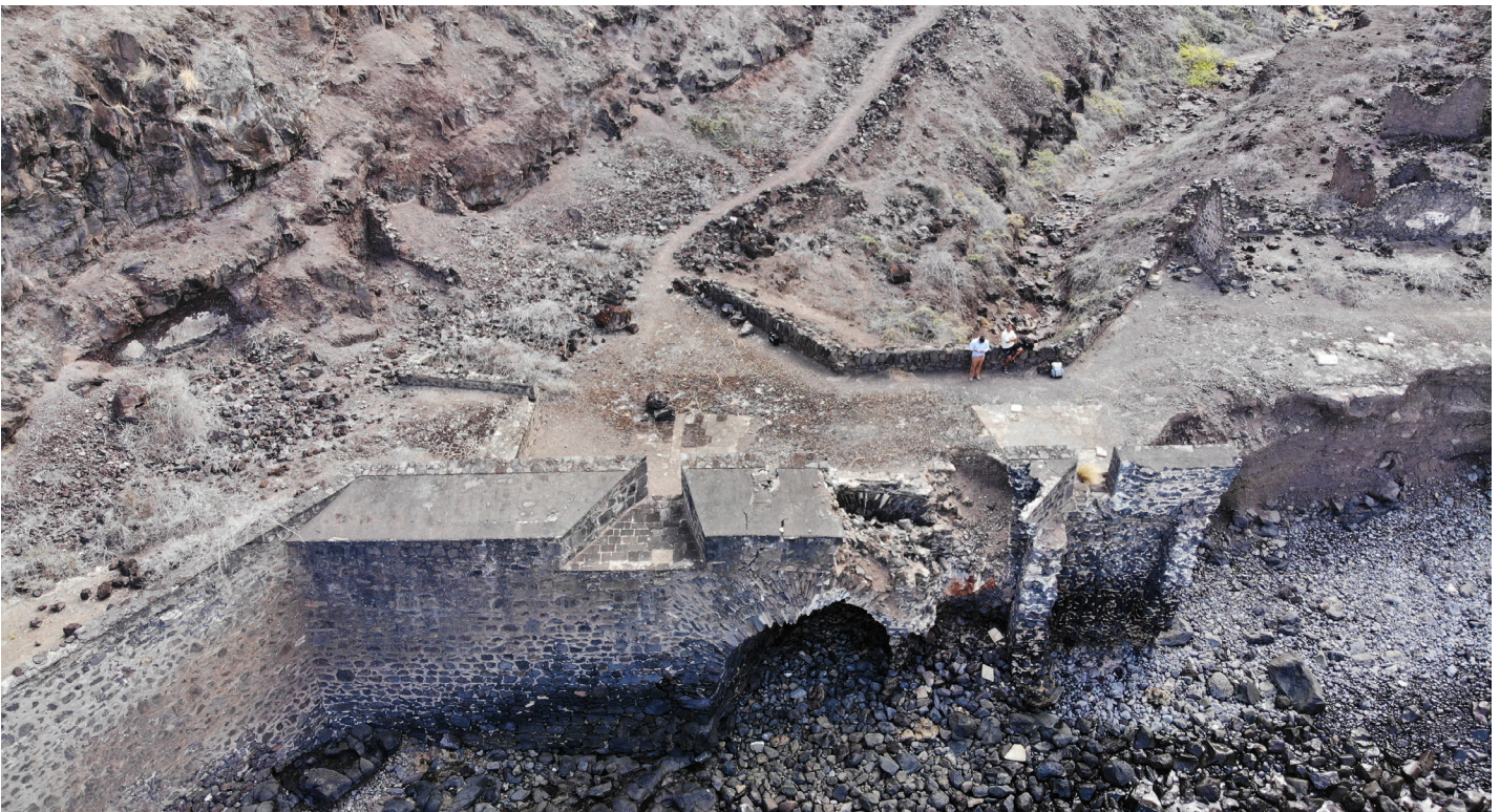
Figure 26: Aerial image of failing curtain wall and support buildings at Lower Banks' Battery (Image: B. Fortenberry).
