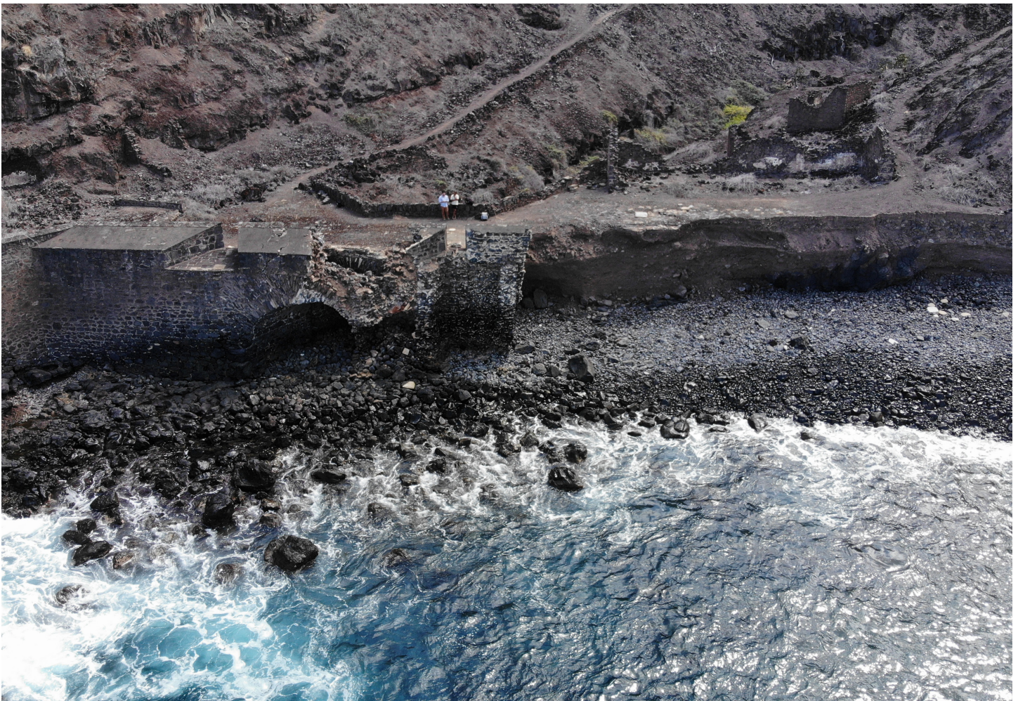
Figure 12: Aerial image with failing Lower Bank's Battery visible (Image: B. Fortenberry).
