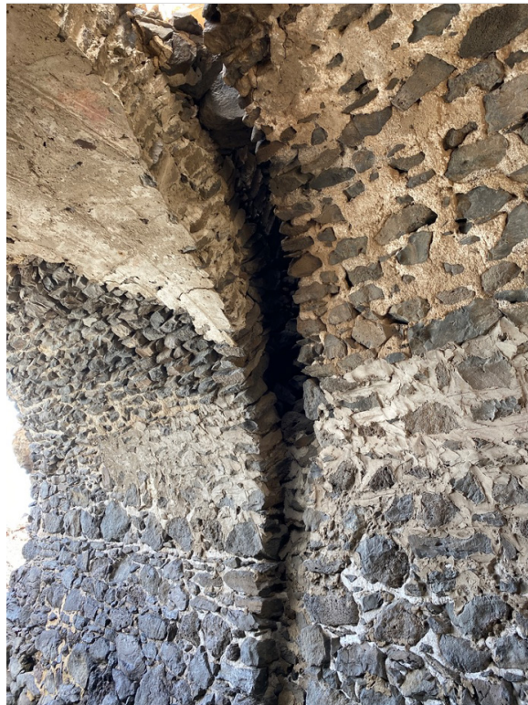
Figure 34: Detail of failing arch at Lower Banks' Battery (Image: B. Fortenberry).
