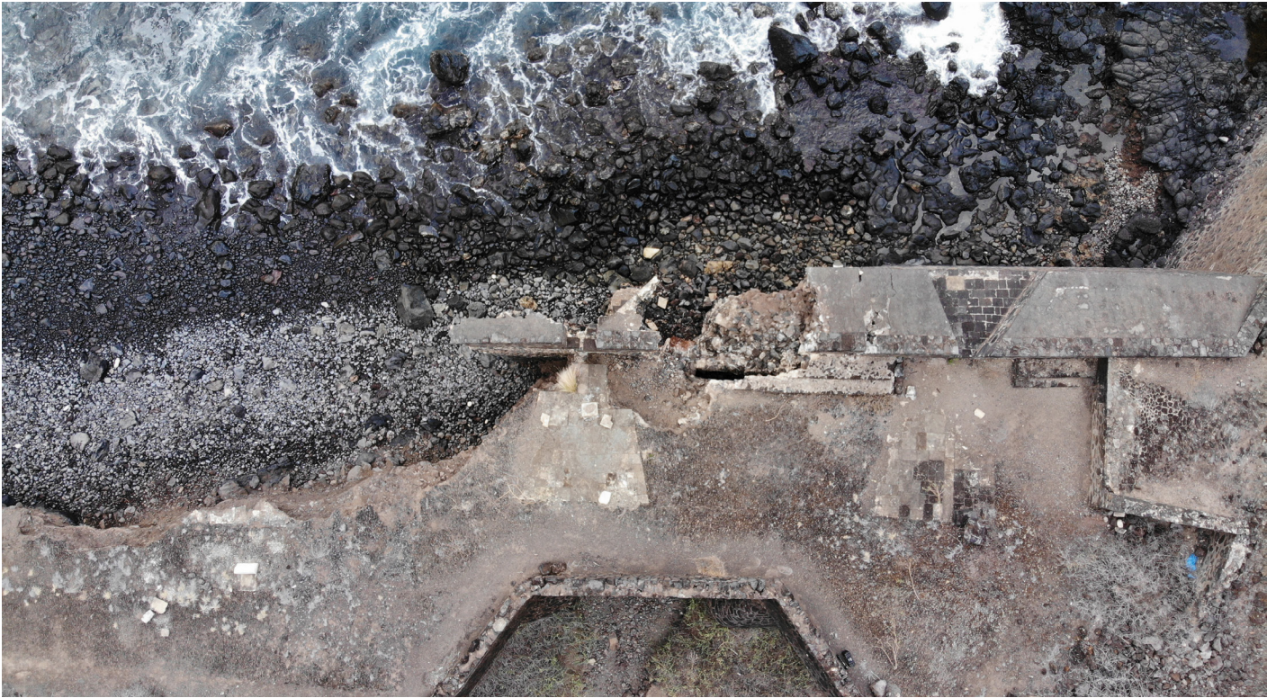
Figure 17: Aerial nadir image of failing curtain wall at Lower Banks' Battery (Image: B. Fortenberry).
