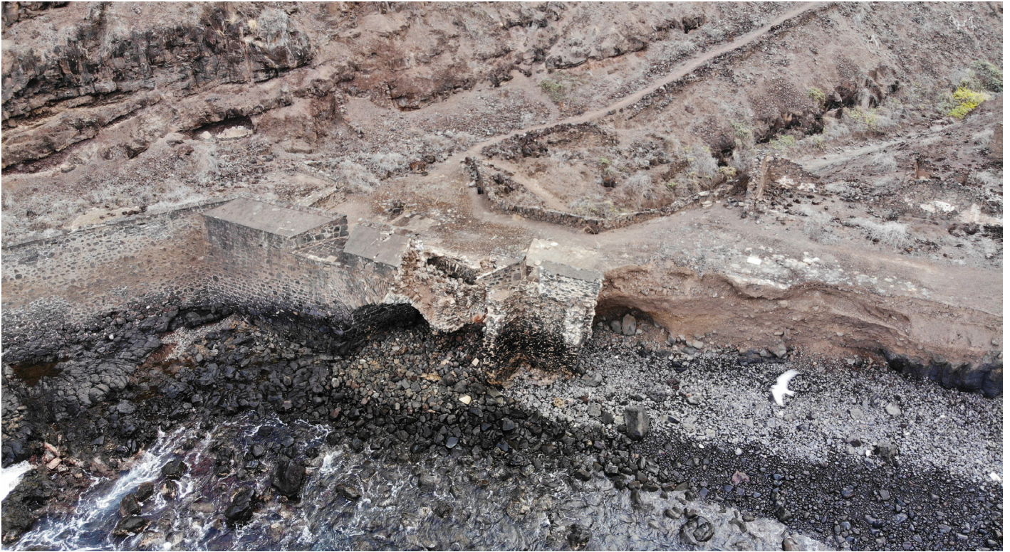
Figure 21: Aerial image of failing curtain wall looking east at Lower Banks' Battery (Image: B. Fortenberry).
