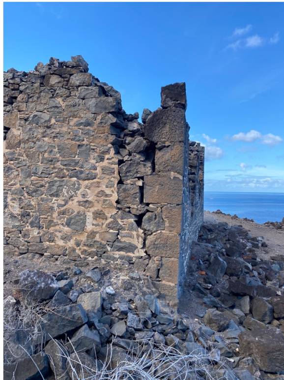
Figure 57: Wall corner collapse at support structure at Upper Banks' Battery (Image: B. Fortenberry).
