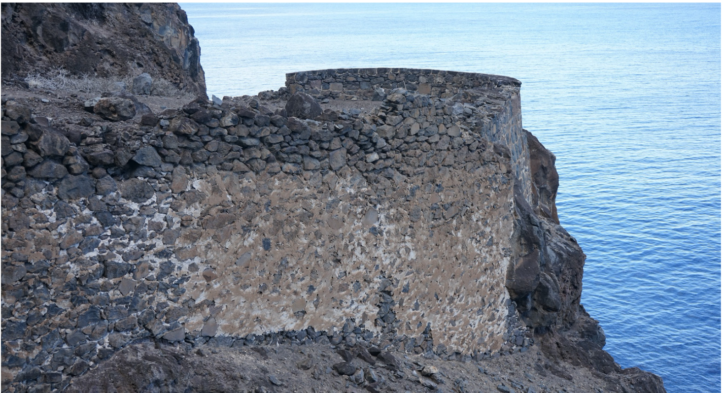
Figure 53: Historically repaired wall on the north edge of Half Moon Battery at Upper Banks' (Image: B. Fortenberry).
