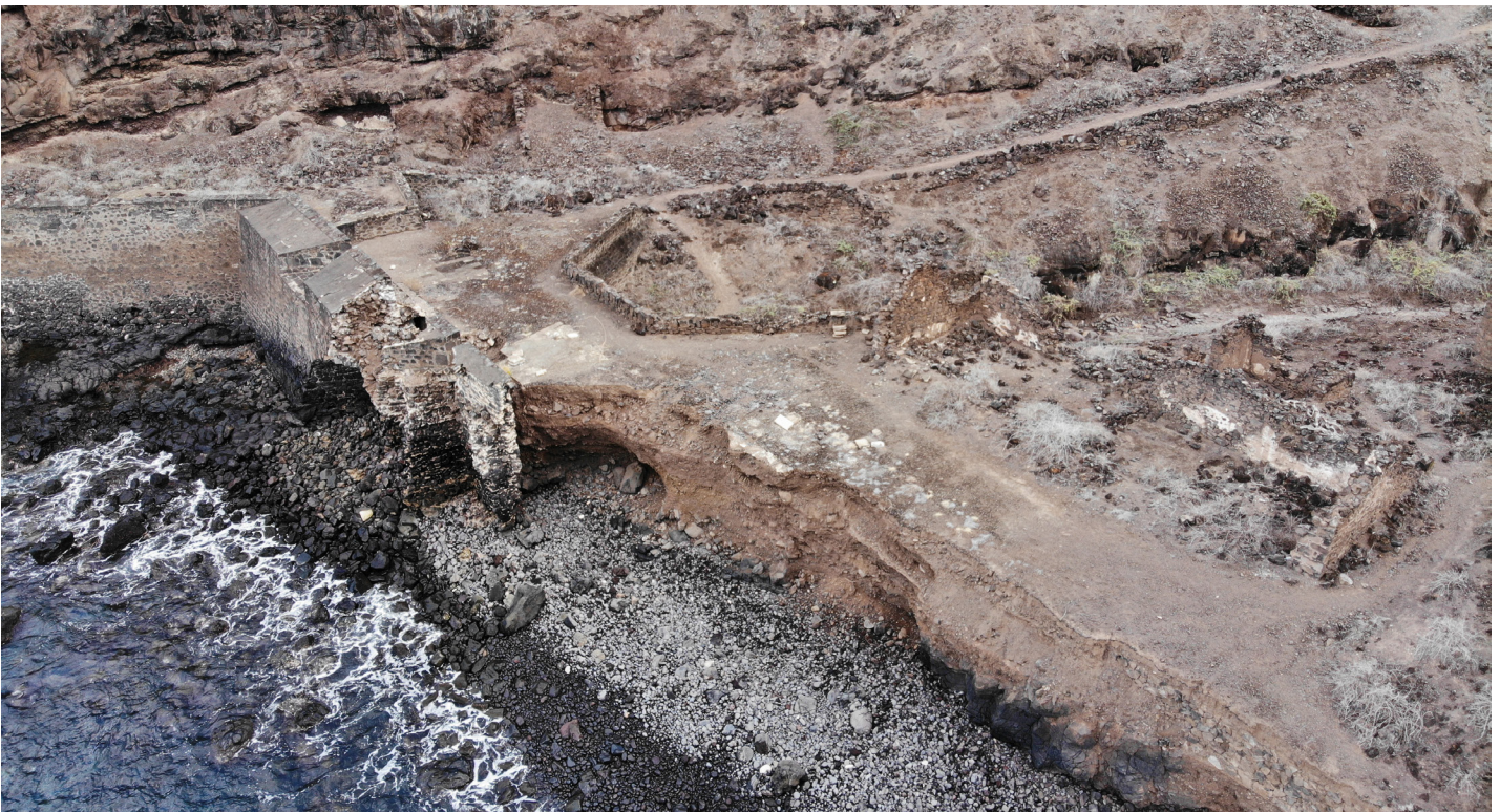
Figure 20: Aerial image of failing curtain wall and lost rampart Lower Banks' Battery (Image: B. Fortenberry).
