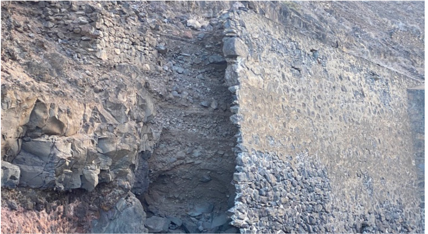
Figure 31: Detail image of northern failure of north curtain wall at Lower Banks' Battery (Image: B. Fortenberry).
