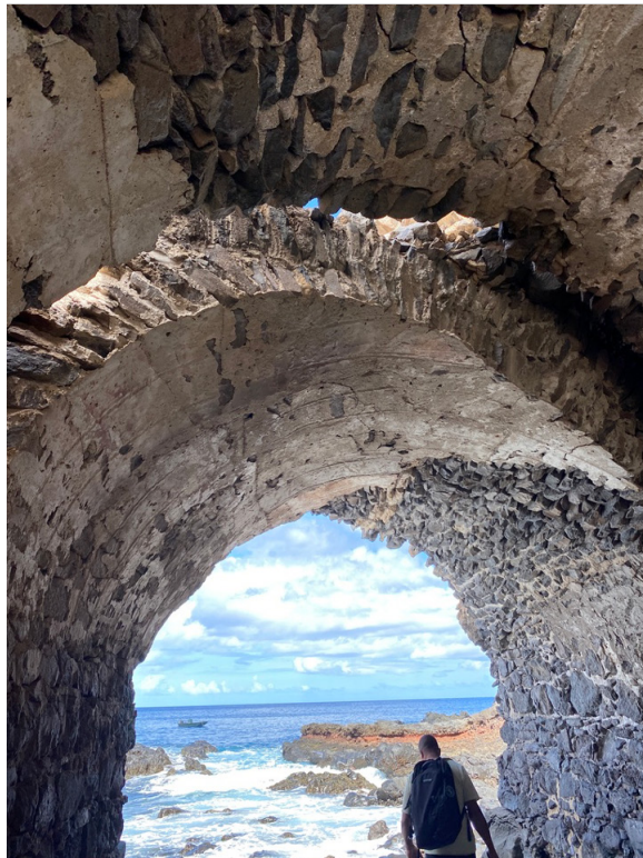
Figure 32: Detail of failing arch at Lower Banks' Battery (Image: B. Fortenberry).
