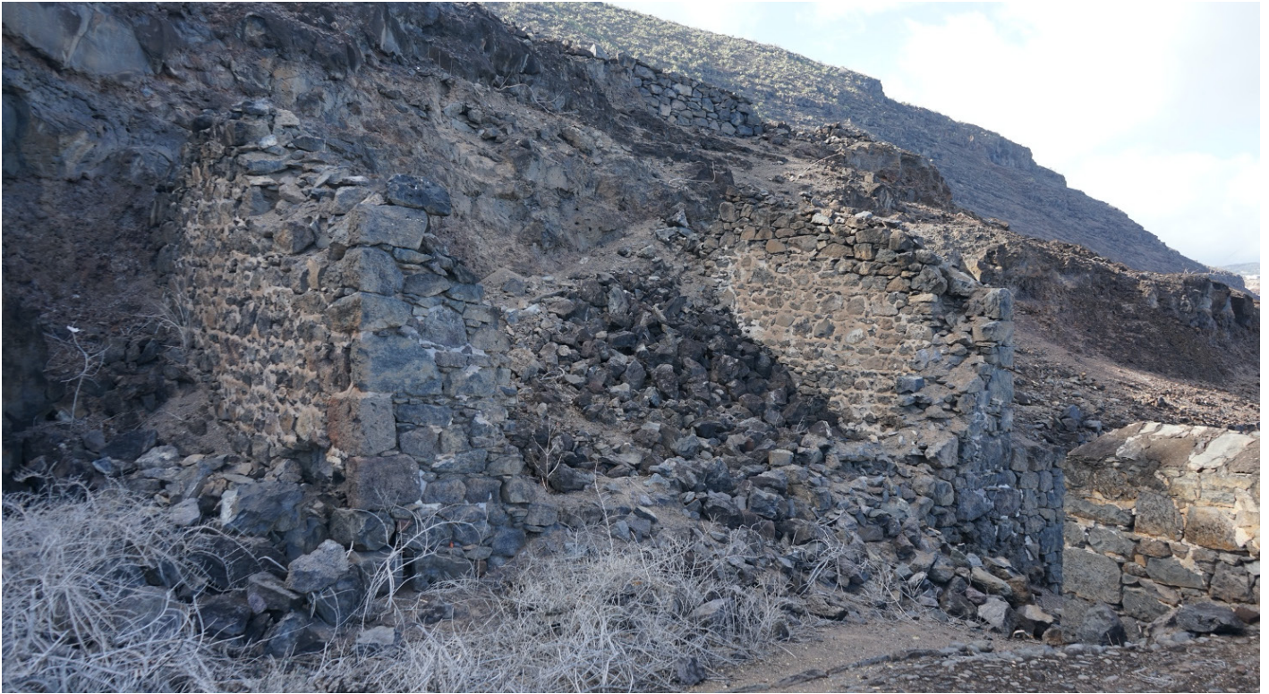
Figure 54: Collapsed support structure on the north edge of Half Moon Battery at Upper Banks' (Image: B. Fortenberry).
