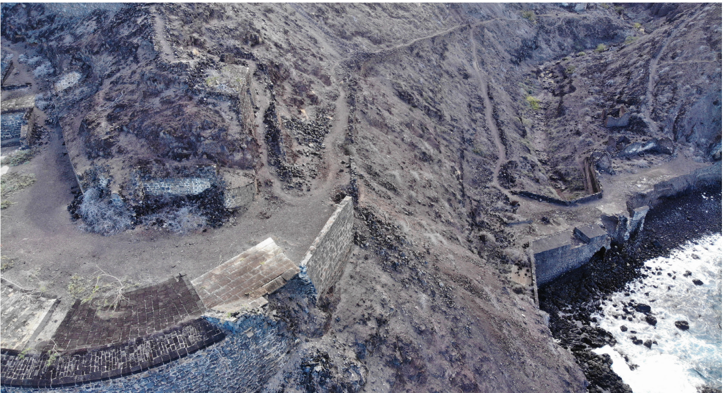
Figure 47: Oblique aerial view of ruined structures and wall collapse at Upper Banks' (Image: B. Fortenberry).
