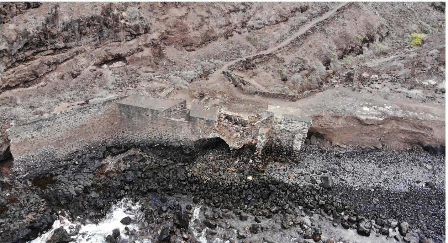
Figure 22: Aerial image of failing north wall and curtain wall at Lower Banks' Battery (Image: B. Fortenberry).
