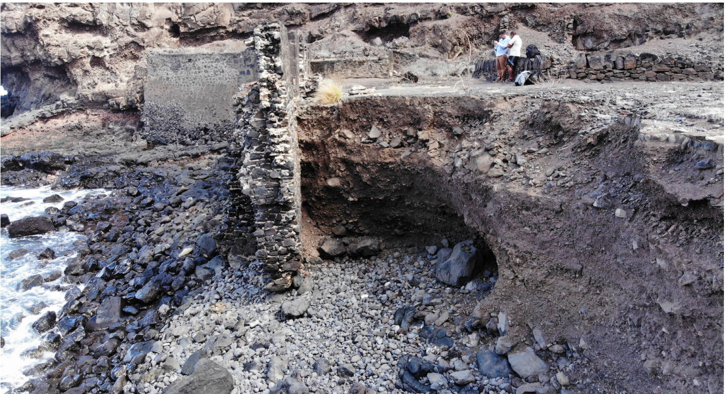
Figure 30: Detail section view of failing curtain wall at Lower Banks' Battery (Image: B. Fortenberry).
