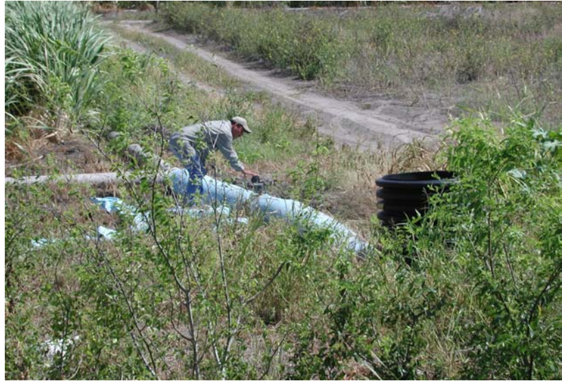
Figure 8. Recording flows with in-line saddle propeller meter.
