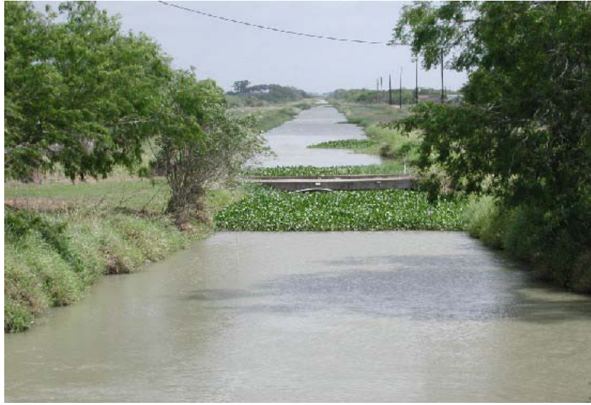
Figure 2. Culvert clogged by aquatic vegetation (Water Hyacinth)
