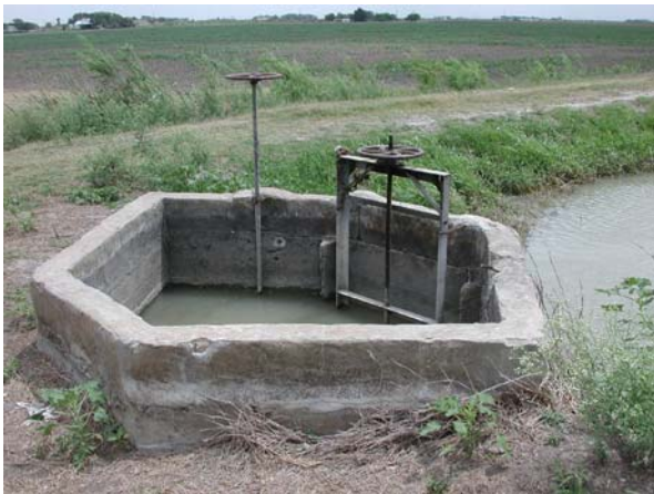
Figure 9. A box head gate situation that typical occurs at the beginning of a canal or after a road crossing. This controls downstream, levels and supplies usually two farm turnouts.
