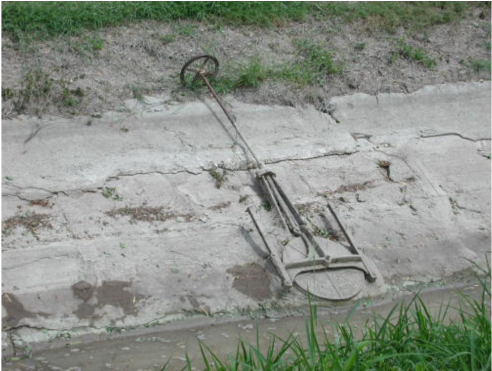
Figure 8: Cracking of lateral A - Stewart just down stream of the test section.
