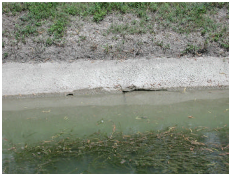
Figure 4: Large crack in the canal lining and aquatic vegetation growing from the bottom of the canal (lateral A - Stewart Rd)
