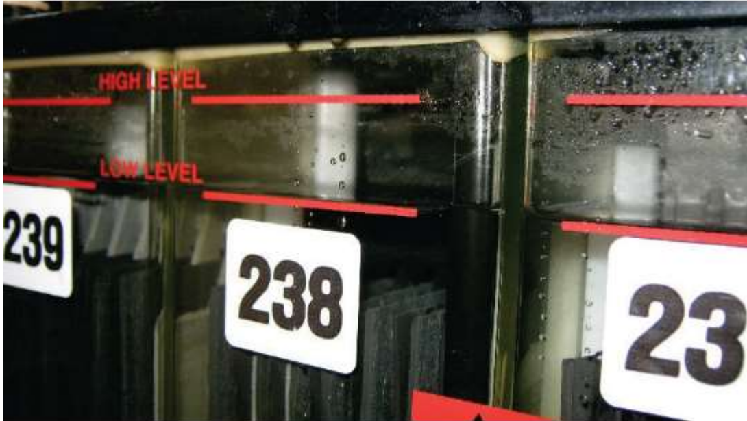
Figure 2.1 Battery with Transparent Case Showing Low Electrolyte Level. Reprinted from [26].
