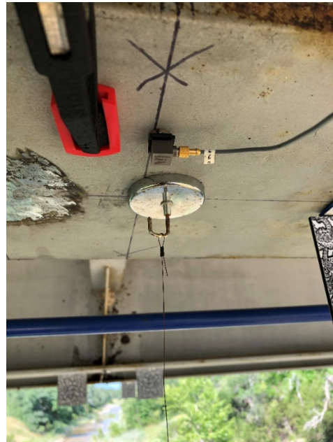
(b) Example of Installed Accelerometer
