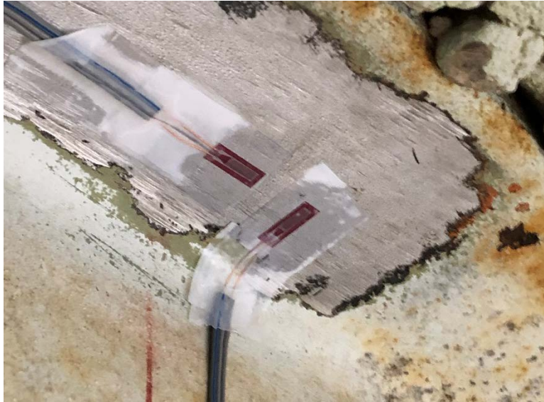
Figure 7.9. Close-Up of Strain Gauge Installation
