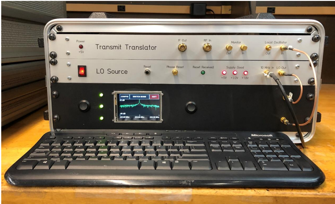
Figure 3.2: Equipment room frequency translation rack. Units are, from top to bottom: Transmit translation stage, LO source, and power supplies and LO control and monitoring. The touchscreen in the monitoring unit shows the LO output being monitored with FreqShow.
