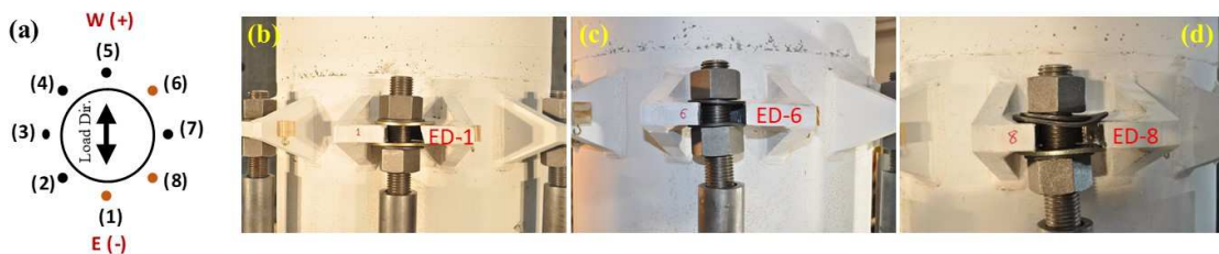
Figure 7.51. Washers deformed in top connection of ED links in PUED rocking column at 1.2 \times DE : (a) location of ED links with deformed washers (brown circles); (b) ED-1; (c) ED-6; (d) ED-8.
