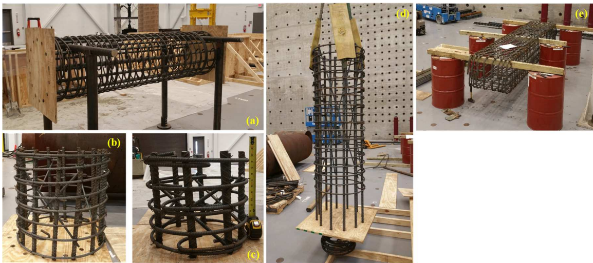
Figure 7.19. Reinforcement cages: (a) RC rocking column; (b) PT anchorage block; (c) central core of PU bi-layered segment; (d) RC segment with steel collar; (e) cap beam.
