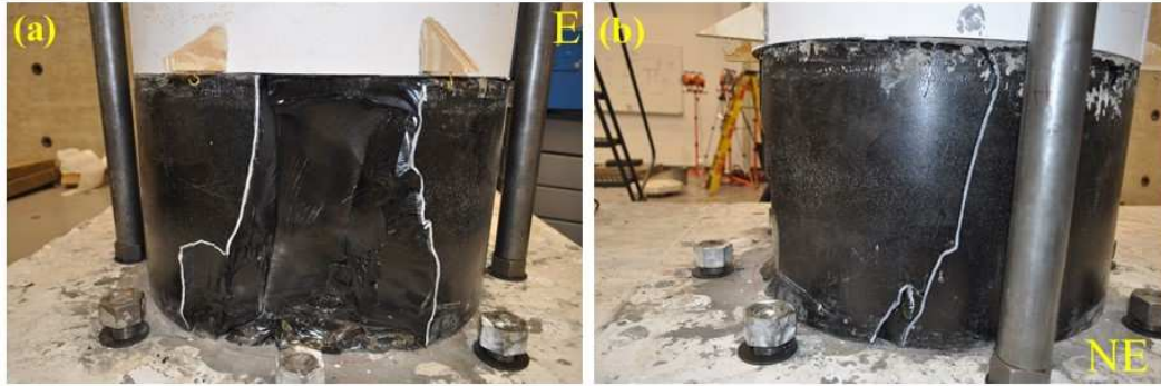
Figure 7.71. Damage state in PUED-2 column at 9.24% drift ratio at the loading rate of 2.71 in/sec (0.025 drift ratio/sec): (a) PU complete fracture on east side; (b) crack in PU on northeast side.
