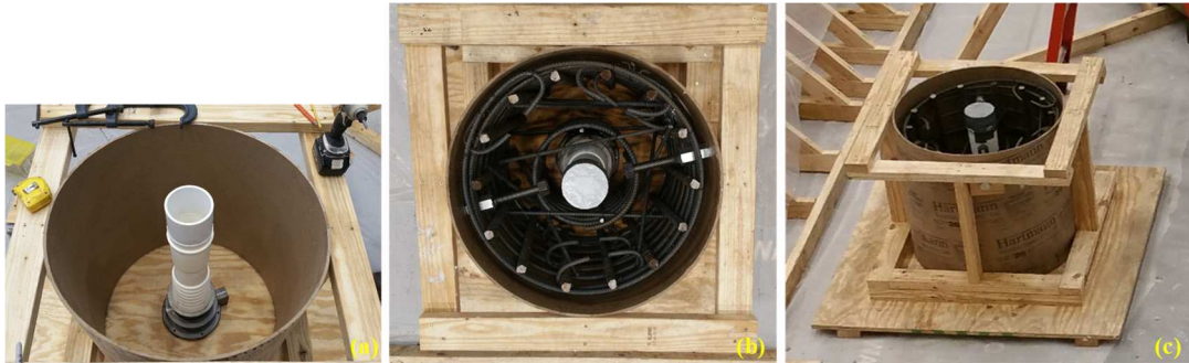
Figure 7.23. Construction steps for PT anchorage block: (a) embedded components of the PT system; (b) top view of the final assembly; (c) isometric view of the final assembly.
