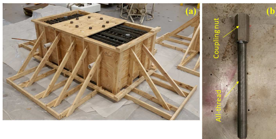
Figure 7.20. (a) Foundation rebar cage in formwork; (b) ED link end anchor setup.
