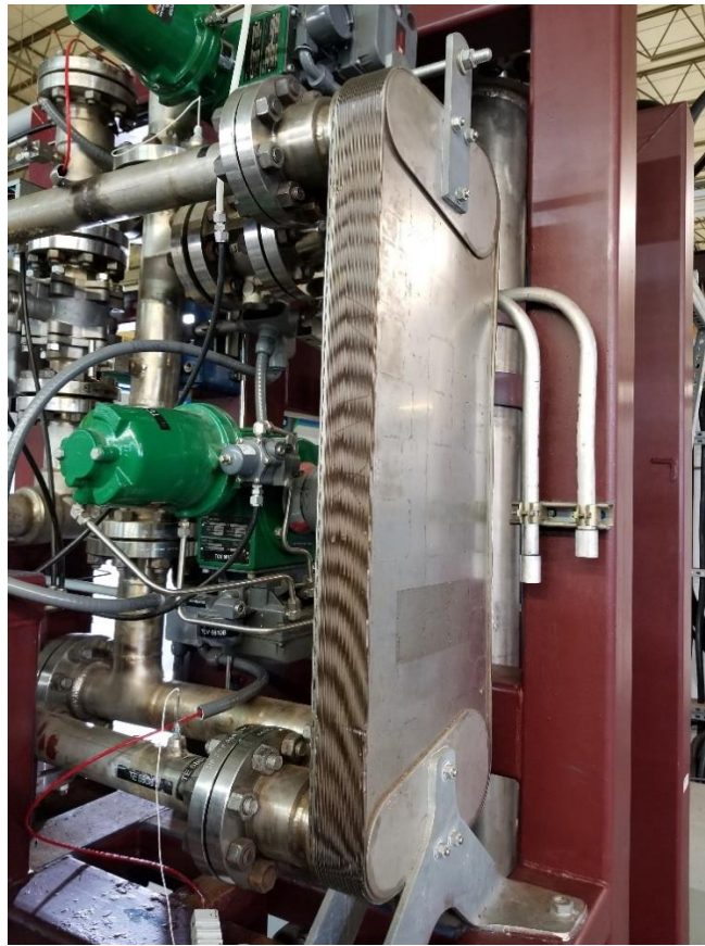
Figure 2.8. Brazed plate heat exchanger which will operate using city water supply.
