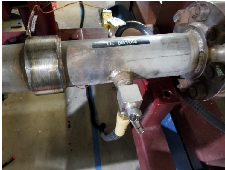
Figure 5.2. Drain valve B near TC5810 G – which is the lowest accessible point in the system.
