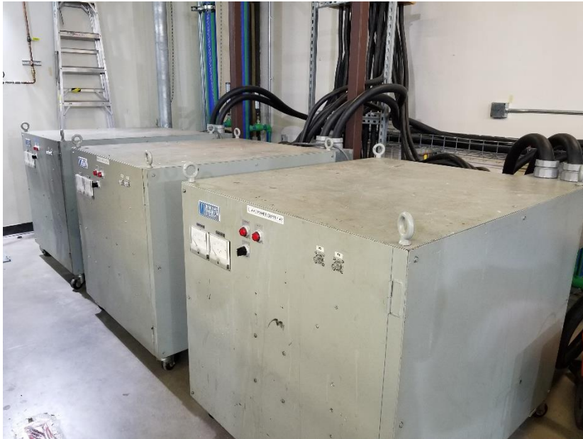
Figure 2.7. Robicon transformers used to convert AC to DC - to electrically heat the rods within the test section.
