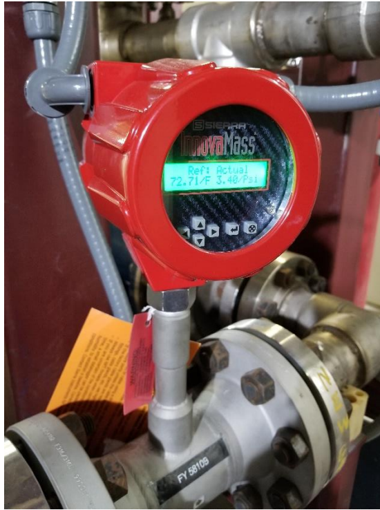
Figure 3.6. Vortex shedding flow meter installed in the primary loop section.
