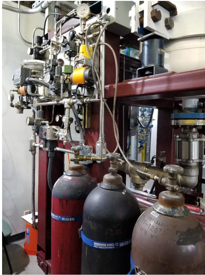
Figure 4.2. Solenoid valves (in orange) along with the pneumatic pressure control valves. The grid is the high-pressure lines carrying compressed air to actuate the valves and N 2 tubing from the tanks, to pressurize the system.
