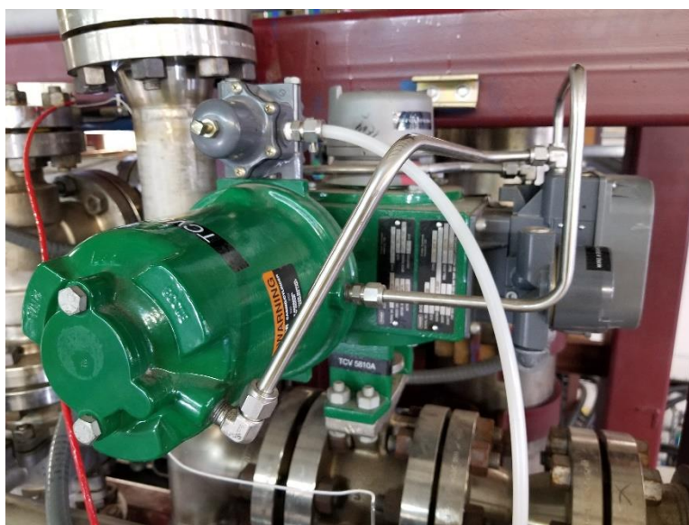
Figure 4.1. Pneumatically operated temperature control valve which regulates flow through the heat exchanger.
