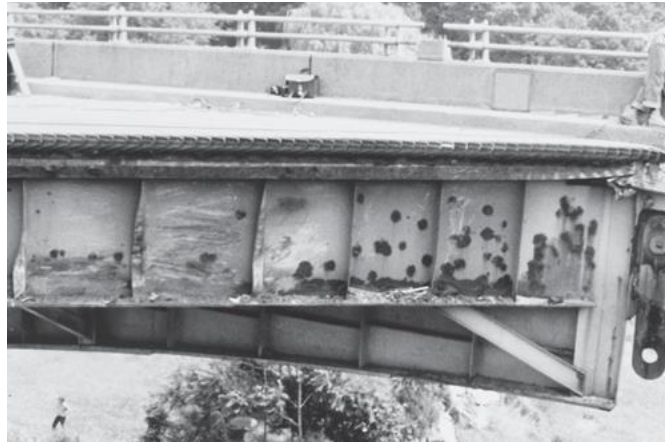
Figure 2.2: Collapse of the Mianus River Bridge (Reprinted from Fisher 1997)
