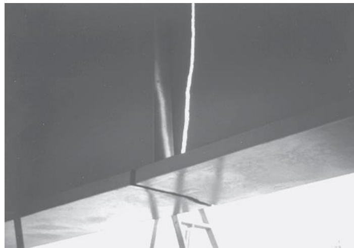
Figure 2.3: Cracked girder of the I-79 Glenfield Bridge in 1977 (Reprinted from Fisher 1984)
