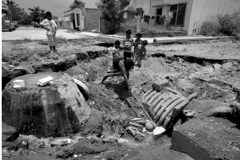
Figure 2.9 Raw sewage near her home in Colinas de Santa Fe in Veracruz, Mexico. Source: Reprinted from the LA Times article “Mexico’s Housing Debacle” by Richard Marosi, 2017. Photography by Brian van der Brug / Los Angeles Times, Marosi, 2017.
