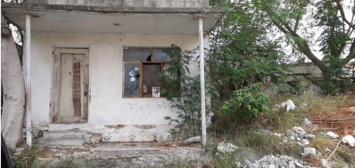
Figure B-1 Own Photographs. Abandoned Housing: Zona Centro, Reynosa, Tamaulipas, Mexico (2019).
