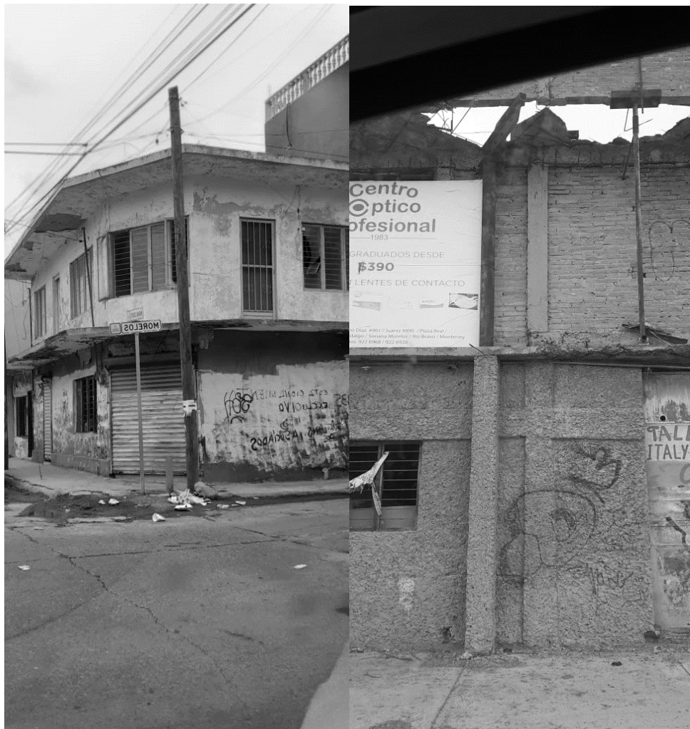
Figure B-4 Own Photographs. Abandoned Housing: Colonia Cañada, Reynosa, Tamaulipas, Mexico (2019).
