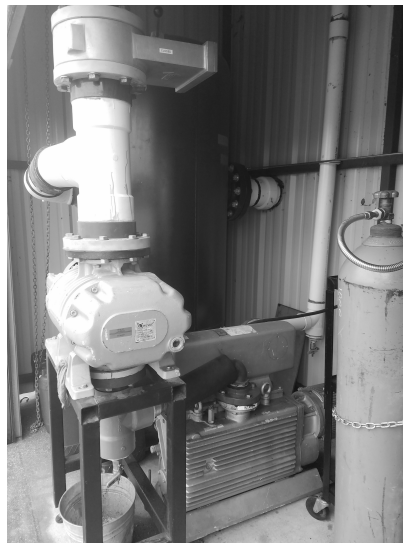
Figure 4.3: Picture of dump tank and vacuum pump infrastructure.
