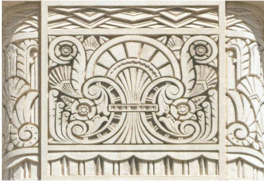
Figure 12. Example of the fan motif on an Art Deco era building. Mark Lemmon, architect, Tower Petroleum Building (detail) , 1931. [18]
