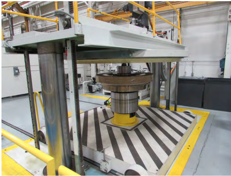
Figure 22: Photo of New Mandrel Assembly Prior to Being Lowered Into The Overspeed Pit
