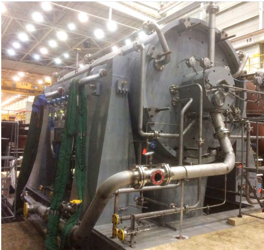
Figure 5: Photo of Compressor
