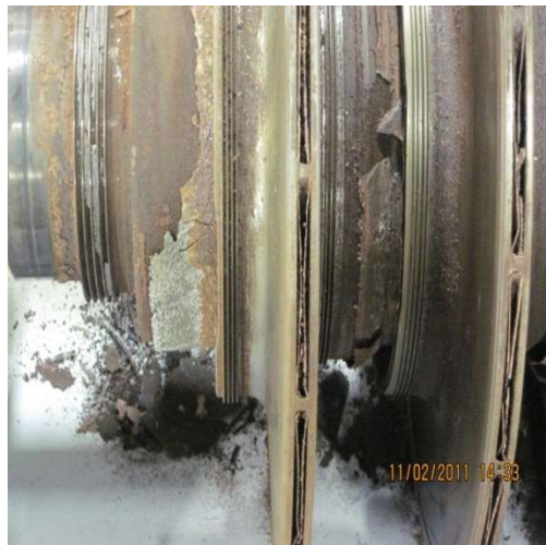
Figure 27: Ammonium Chloride Fouling in a Hydrogen Recycle Compressor
