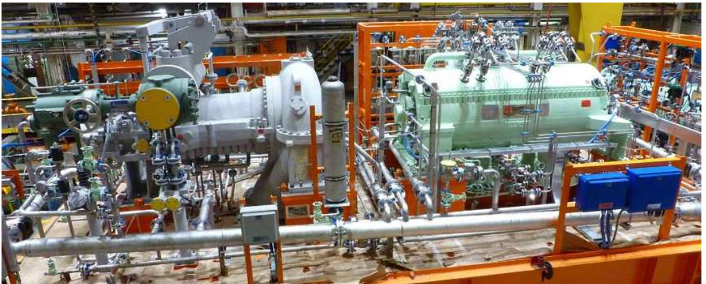
Figure 11: Steam Turbine Driven Wet Gas Coker Compressor
