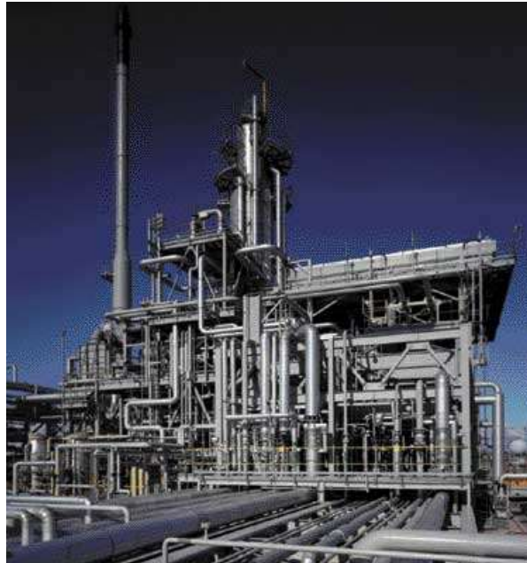
Figure 3: Hydrotreater Unit Grangemouth, UK
