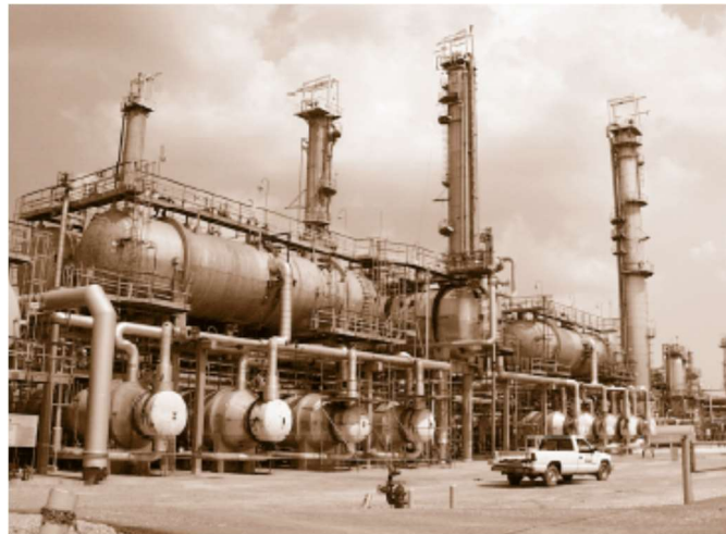
Figure 8: Alkylation Plant (Courtesy of Motiva)
