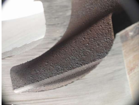
Figure 28: Pitting Corrosion in 17-4 PH Stainless Steel Underneath Foulant Build-up in Figure 27
