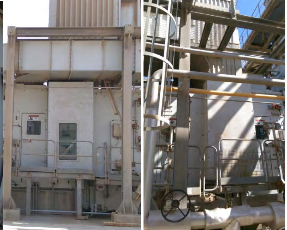
After applying Inlet vertical wall reduction Inlet vertical wall on the back and front side
