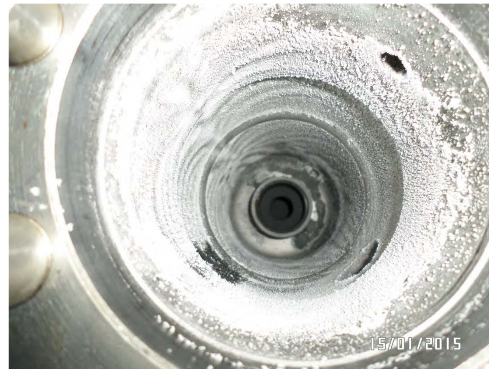
Seal gas filter housing, the clean side
