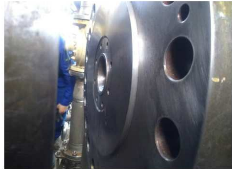
Flanges after cleaning
