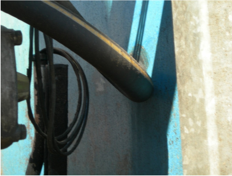
Figure 1b Hose in operation causing wear.
