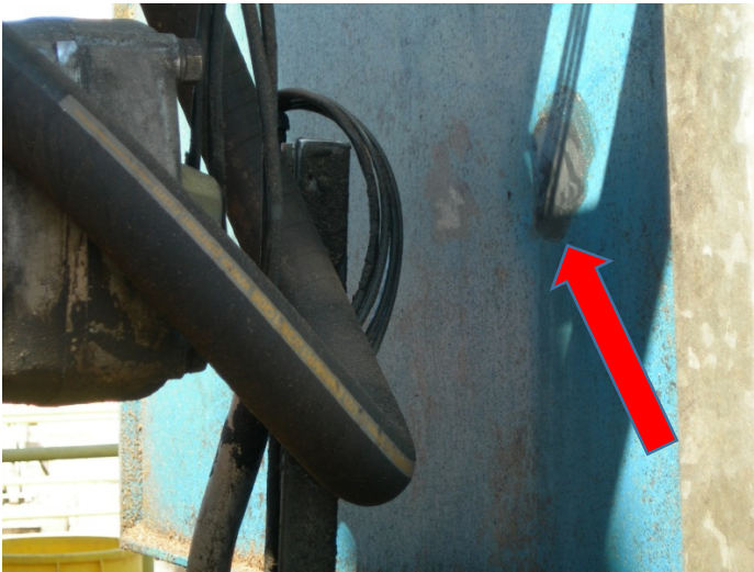
Figure 1a Mark seen on tank during operator rounds
