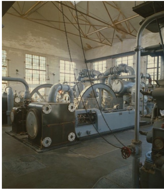
Figure 2: Pumps with flywheels for surge protection.
