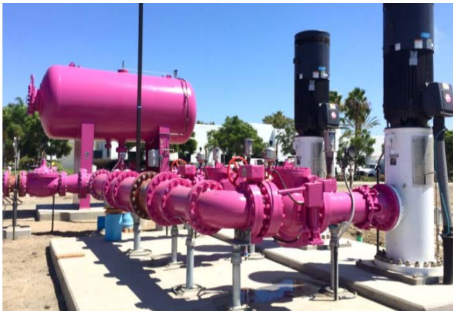
Figure 8: Closed surge vessel at a reused water pump station.
