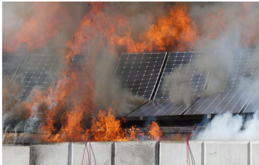
Figure 1. An example of solar PV fires.
