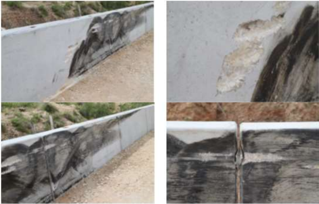
Figure 148 Post-crash views of the barriers from the traffic side
