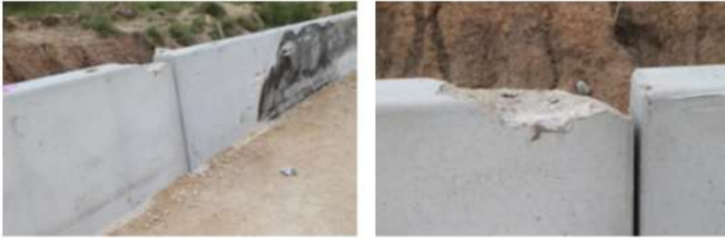
Figure 147 Damage in barrier
