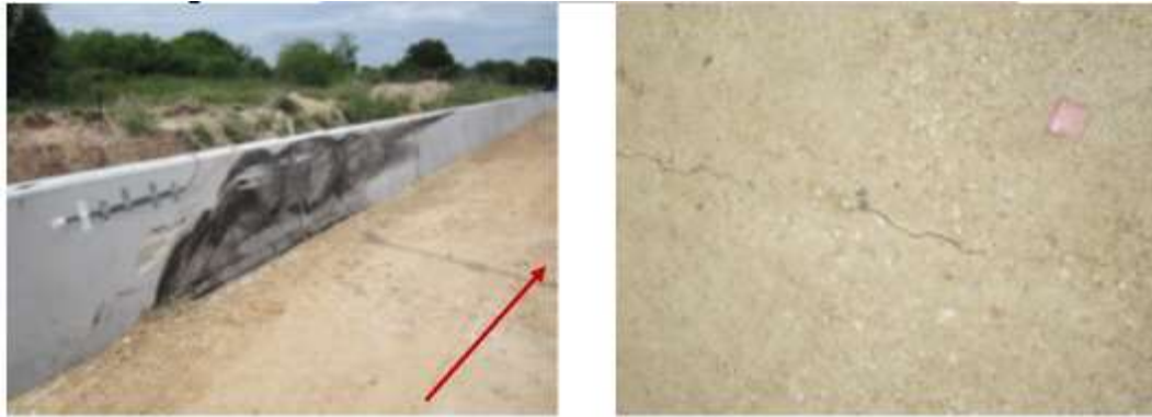
Figure 149 Crack in the compacted fill over the edge of the moment slab
