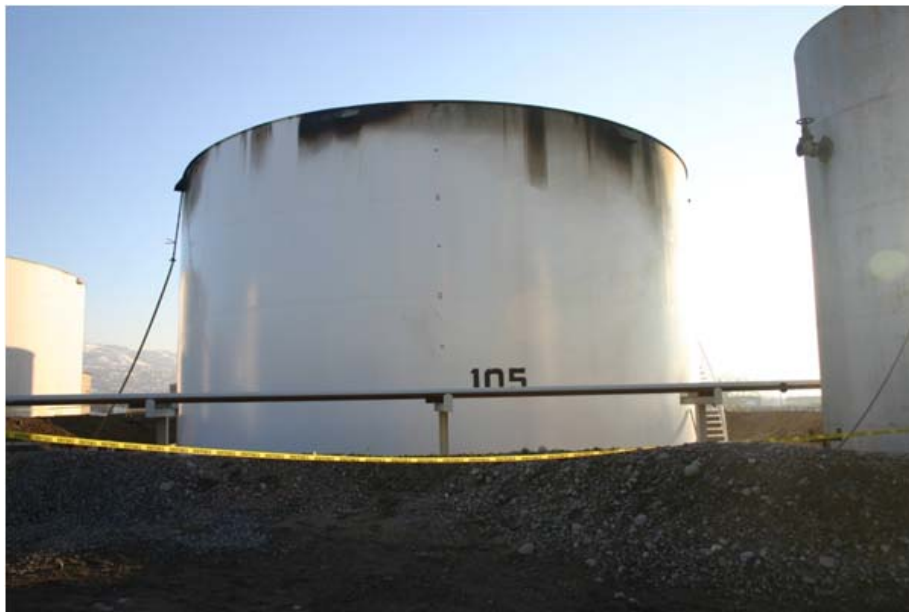
Figure 8: The Tank that Caused Silver Eagle Refinery Flash Fire and Explosion 7
