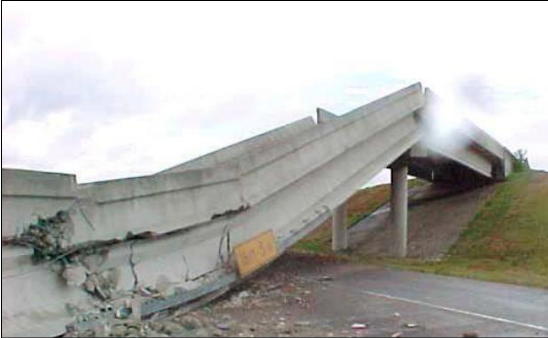
Figure 1. Collapsed Bridge in Dallas, Texas (TxDOT, 2001)
