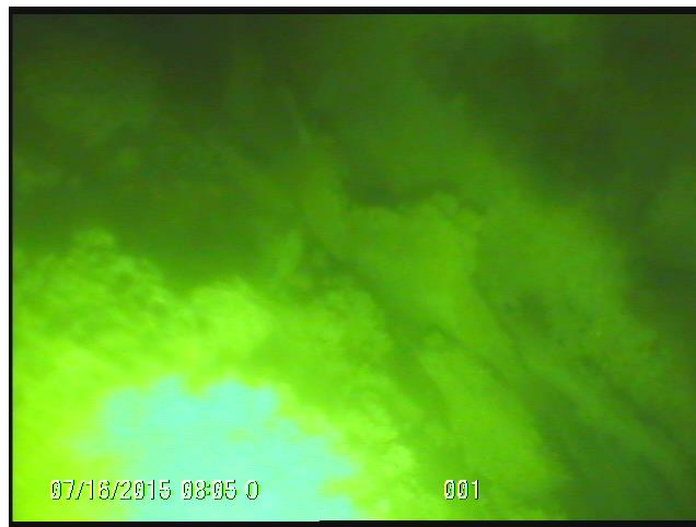
Figure B.6-6: Borescope Photo of Grout Segregation in Specimen 2 Grid H-I
