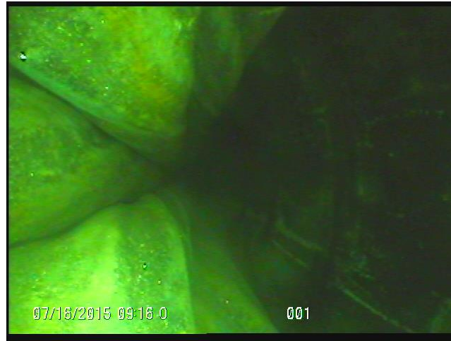
Figure B.6-9: Borescope Photo of Intact Strands in Specimen 4 Grid F-G
