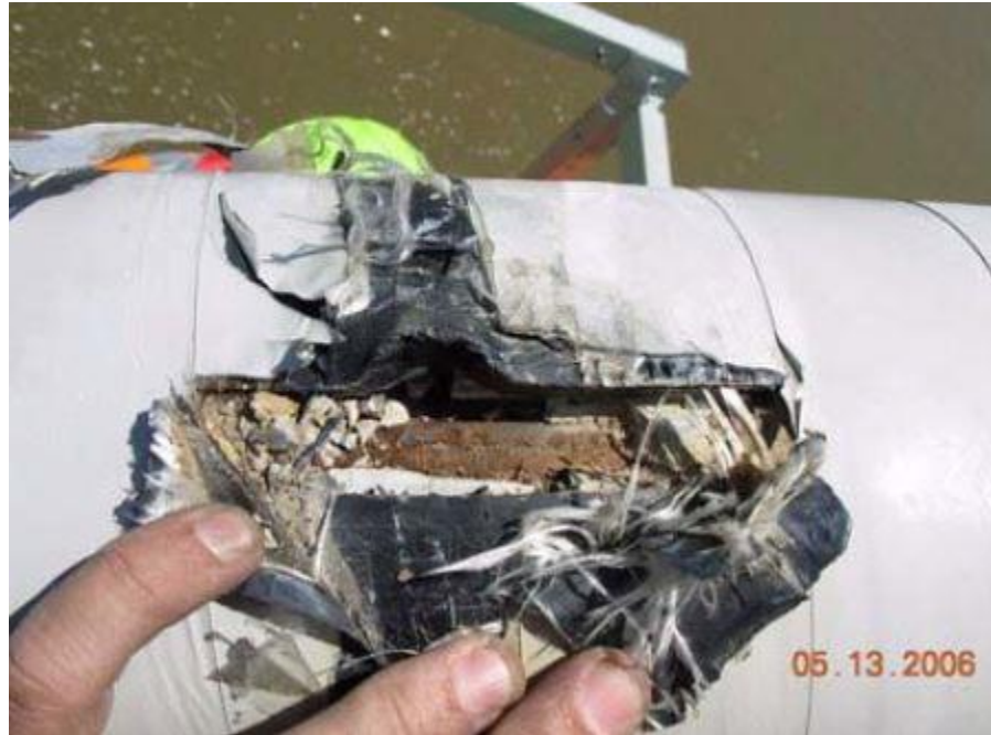
Figure 2-3: Corrosion of steel wires in Luling Bridge stay cable (Mehrabi, 2009)
