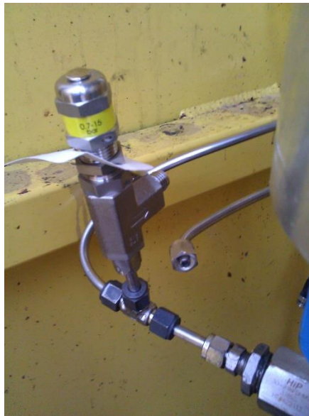
Figure 87: Relief valves mounted to fuel and oxidizer lines.
