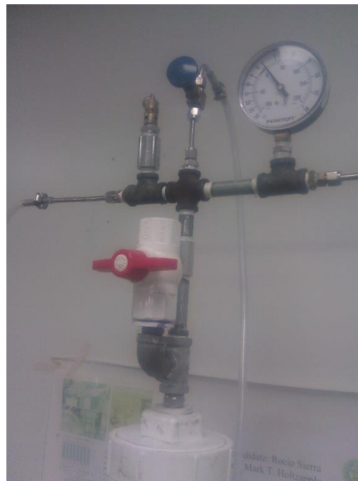
Figure 36: Manifold controlling air flow through CO 2 -scrubbing column.
