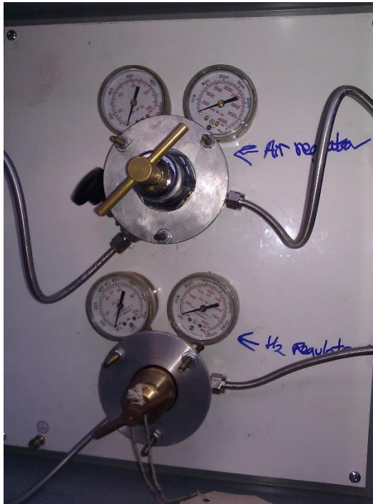
Figure 86: Redundant, step-down regulators mounted to bunker wall.
