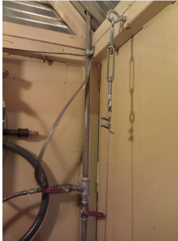
Figure 72: Exhaust pipe and grounding wire.
