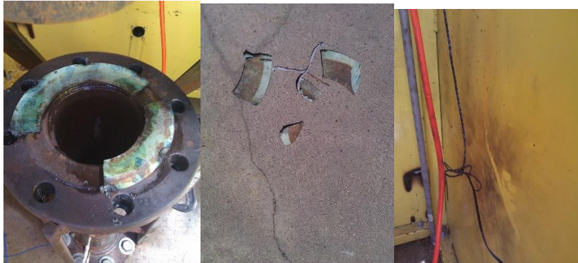
Figure 105: Aftermath of catastrophic gasket failure and blow-out.
