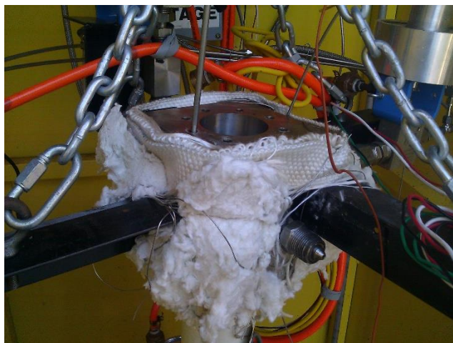
Figure 95: Gas manifold with heating tape applied.
