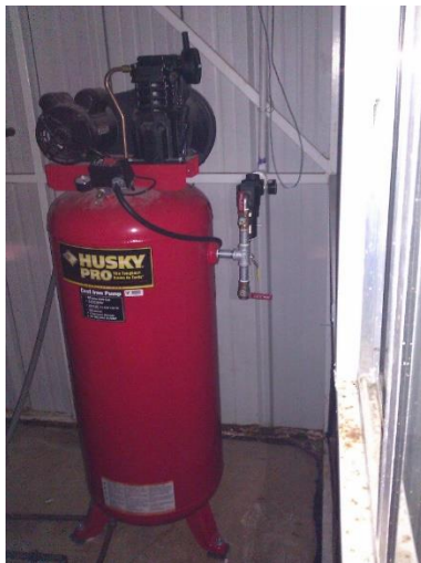
Figure 73: Air compressor mounted to drive pneumatically actuated needle valves.
