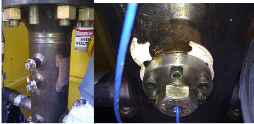
Figure 106: Non-catastrophic failure of Teflon gasket and O-ring seal.
