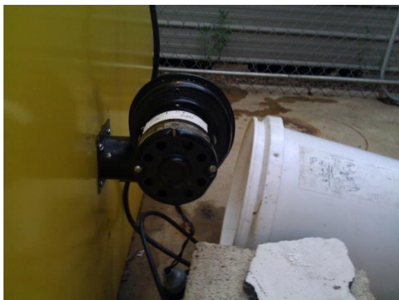
Figure 85: Ventilation blower mounted to bunker wall.
