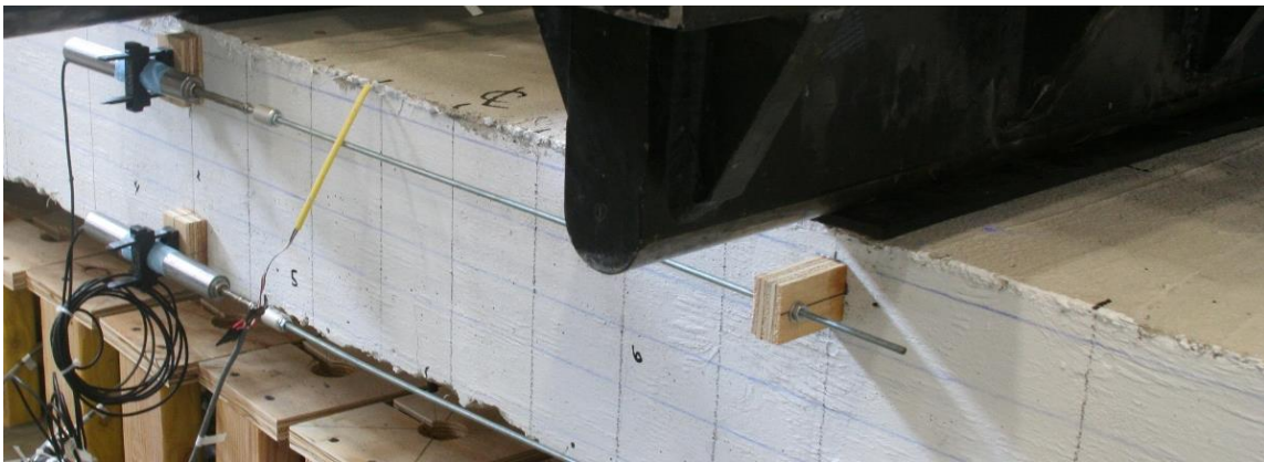
Figure 18. Damaged Corner of S7505BOT24 Where 4 Cracks Have Formed
