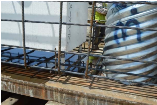
(a) Bottom Cover and Drain Pipes
