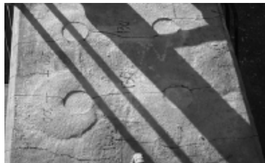
(b) Flexure Cracks at Top of Connection at Max. Realistic Longitudinal Moment
