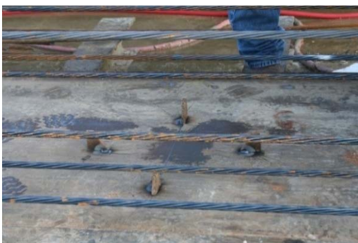
(a) Corrugated Pipe Stumps
