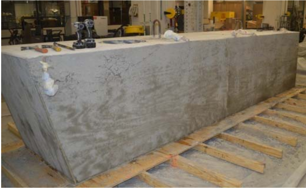
(a) Honeycombing– Front Face of Bent Cap
