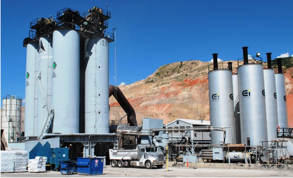
Figure E3. Hot Mix Plant Located at Beck Street Used to Produce PFC Mixture.
