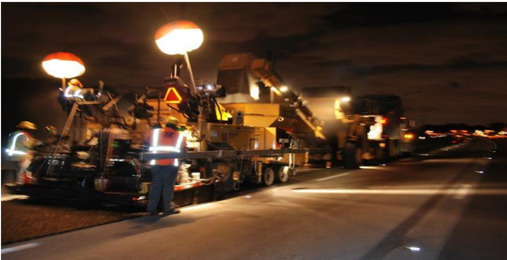
Figure D1. Paving of the OGFC surface course on IH 95 in Florida.
