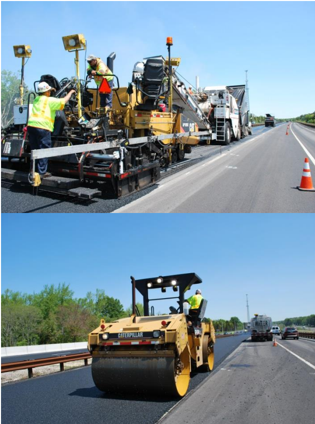
Figure F9. Paving of Friction Course on Garden State Parkway in New Jersey.
