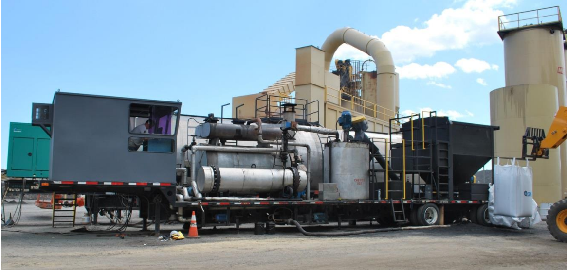
Figure F4. Portable Crumb-Rubber Blending Plant.
