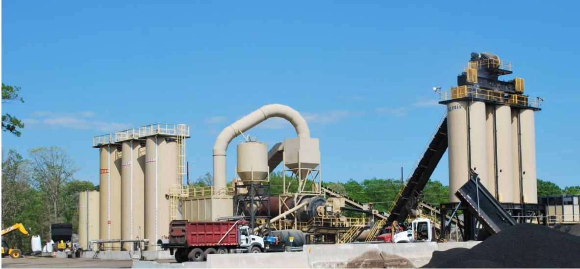
Figure F5. Hot Mix Plant Located at Woodbine, New Jersey.
