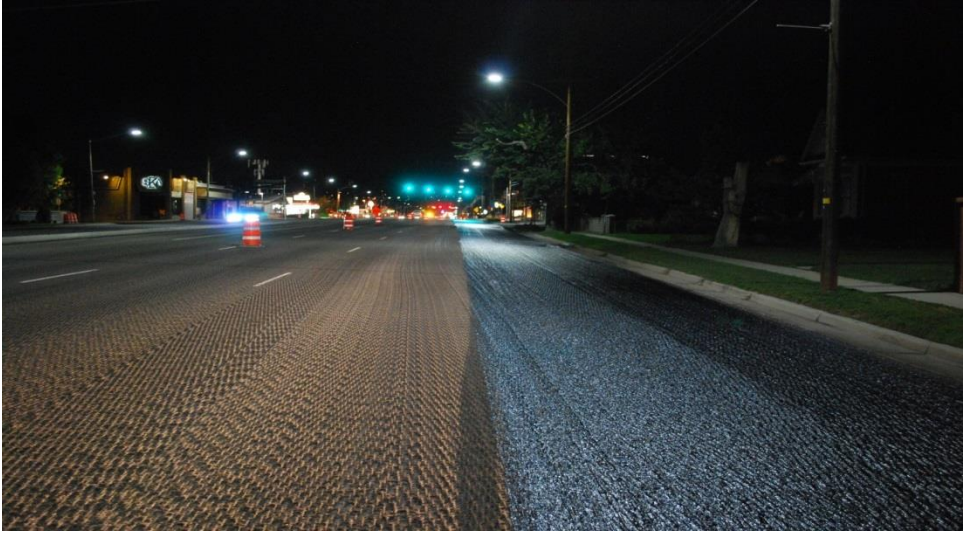
Figure E4. Milled Surface and Tack Application before Paving on SR 71 in Utah.
