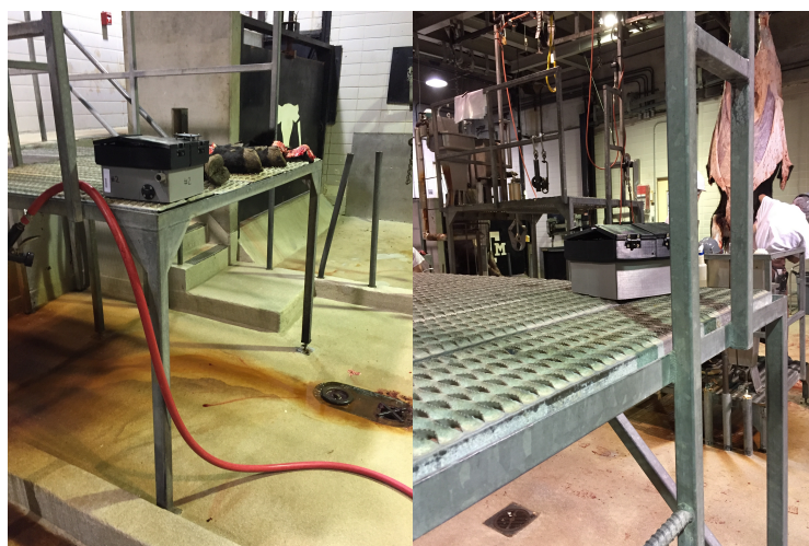
Figure 3: Front of Facility A. (Left) WWC near the bleeding pit. (Right) WWC near the de-limbing area.
