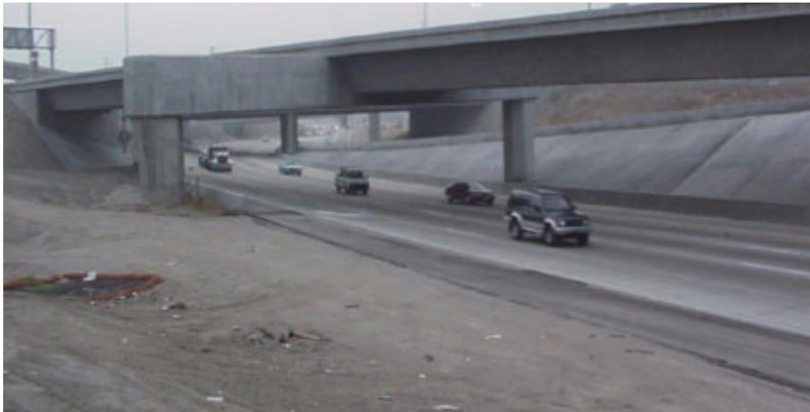
Fig. 4.3: Highway 91/5 over-crossing, located in Orange County- CA, reprinted from Agrawal et al. (2009).
