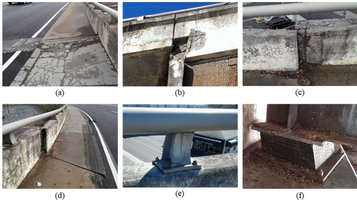
Figure 26: Evidence of Deterioration: a) Cracking along concrete sidewalk, b) Section loss at abutment, c) Spalling on barrier, d) Lateral displacement of barrier, e) Deformed guardrail support, and f) Extended neoprene bearing (Reprinted from Murphy and Yarnold 2018)
