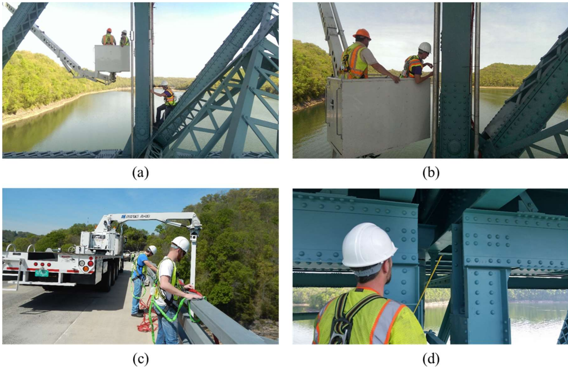
Figure 79: Installation Photos: a) Gage Cable Securement and Installation of Strain Gage on Vertical Member, b) Strain Gage Installation on Catch System, c) Cable Assistance from Bridge Deck, and d) Displacement Gage Installation
